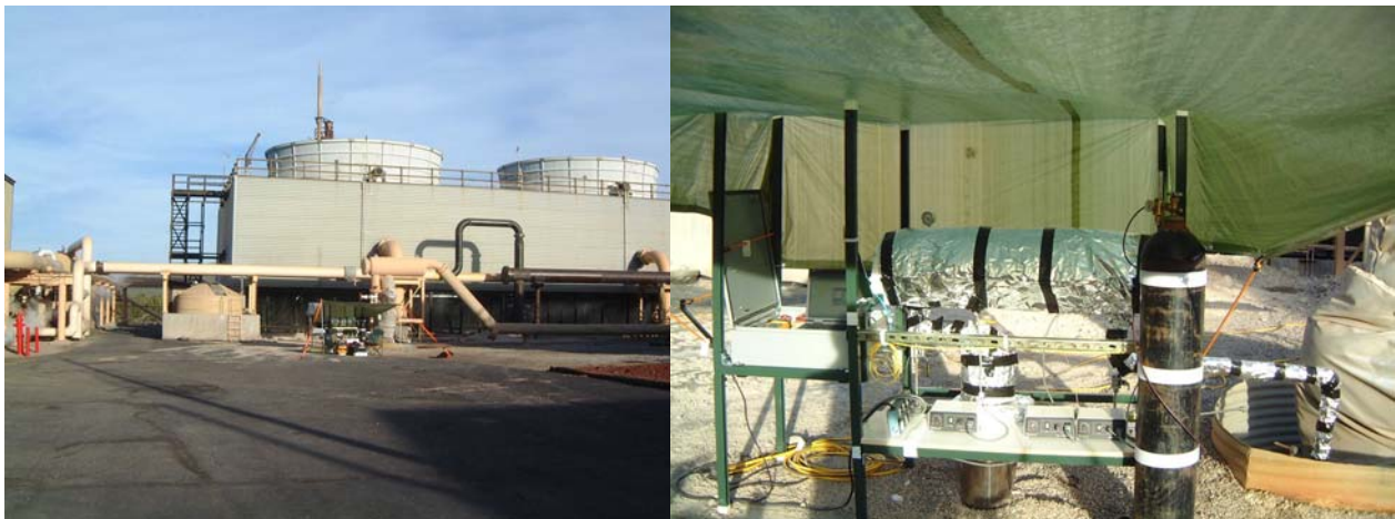
Figure 1. Well Head Installation of the Steam Quality Monitoring Instrumentation at Bonnett Geothermal Plant.
