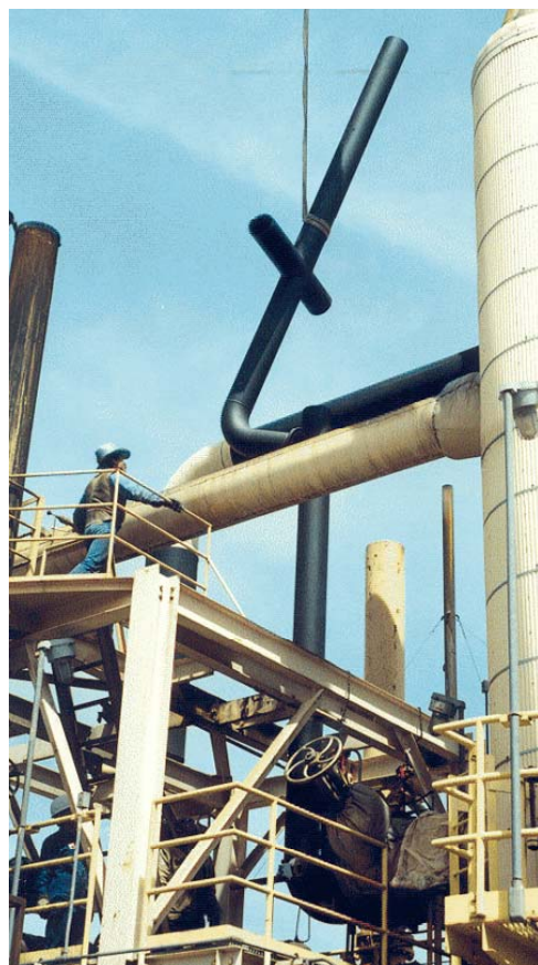
Figure 1. PPS-coated steam vent pipelines being installed at the Cove Fort geothermal plant.
