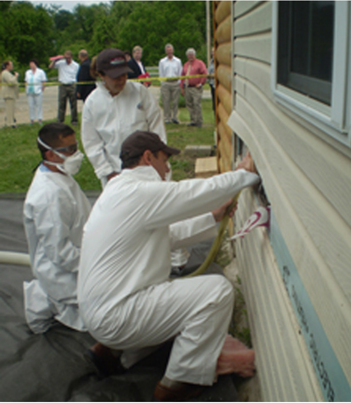
Crew Member Garrett Feaster, one of 15 new crew members at LEADS funded by the Recovery Act, teaches Congressman Zack Space and Ohio Department of Development Director Lisa Patt-McDaniel how to insulate a sidewall on a 100-year-old home in Newark, Ohio. | Photo courtesy Ohio Association of Community Action Agencies
