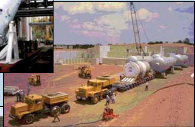
Left: steam generator removal. Below: reactor vessel and large component shipments ready for burial in Barnwell.
