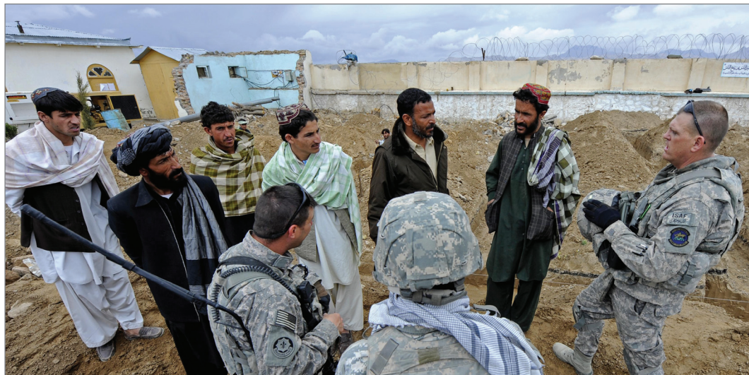
Provincial Reconstruction Team members with Afghan contractors at hospital expansion site. (U.S. Air Force photo)
