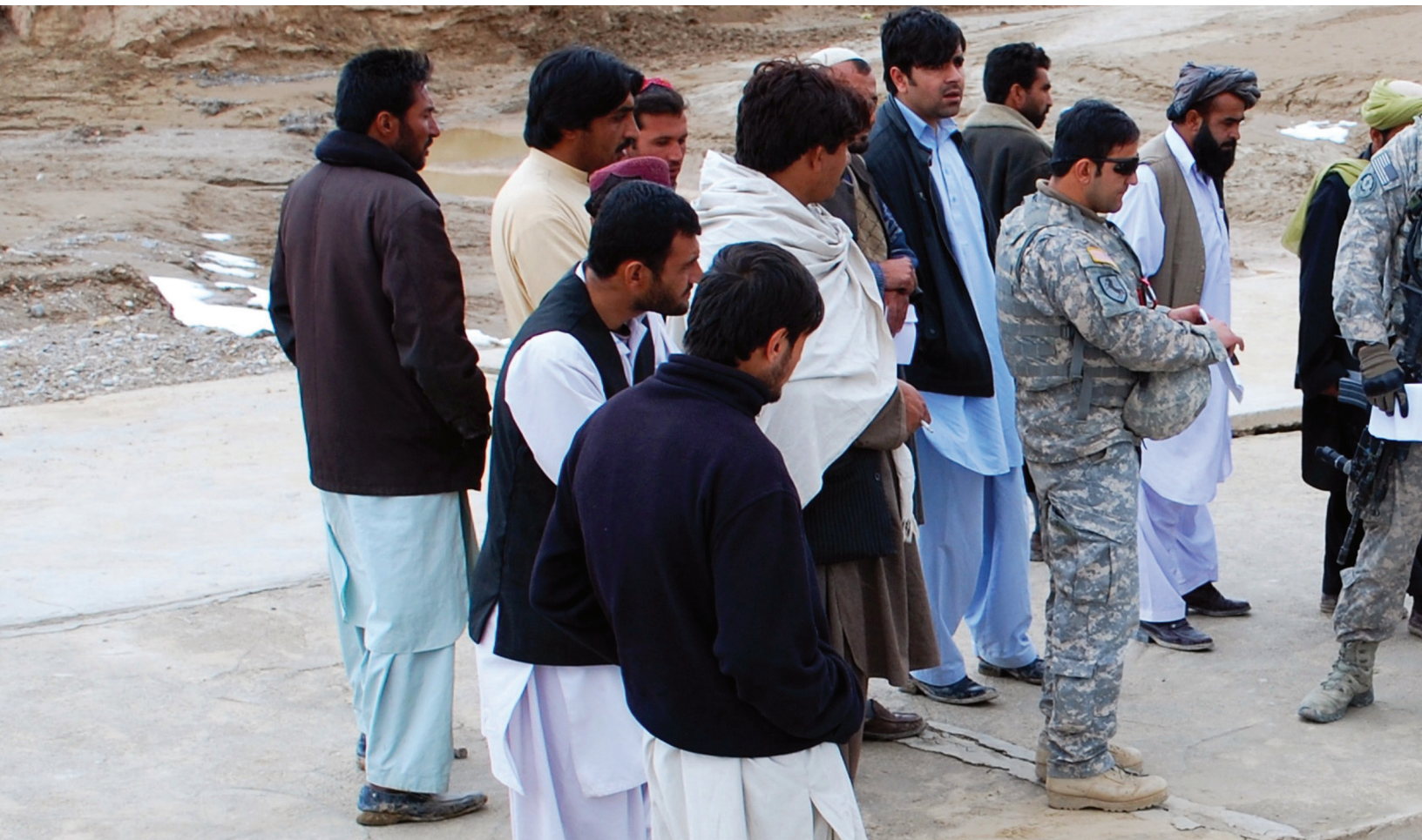
Provincial Reconstruction Team with contractors at bridge-repair job site, Zabol province, Afghanistan. (U.S. Air Force photo)
