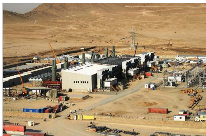
Kabul Power Plant, Afghanistan, 2010. (SIGAR photo)
