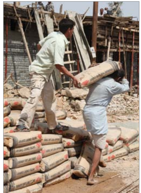
Local contractors at school construction site near Mahmudiyah, Iraq. (U.S. Army photo)
