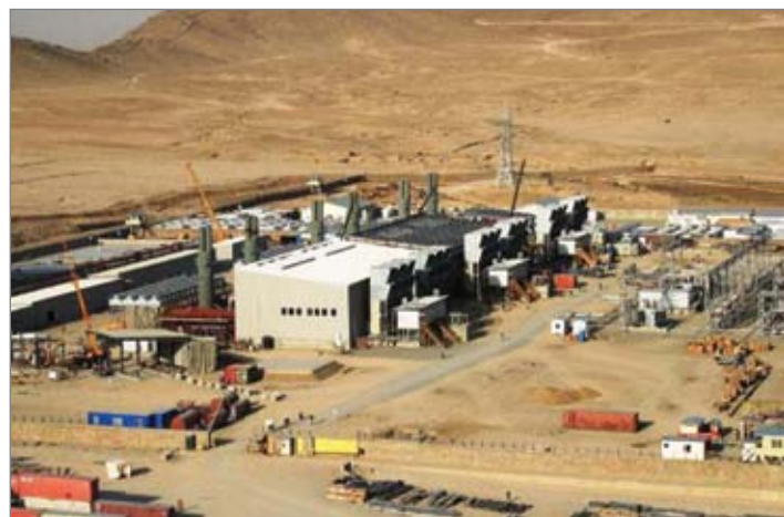
Kabul Power Plant, Afghanistan, 2010. (SIGAR photo)
