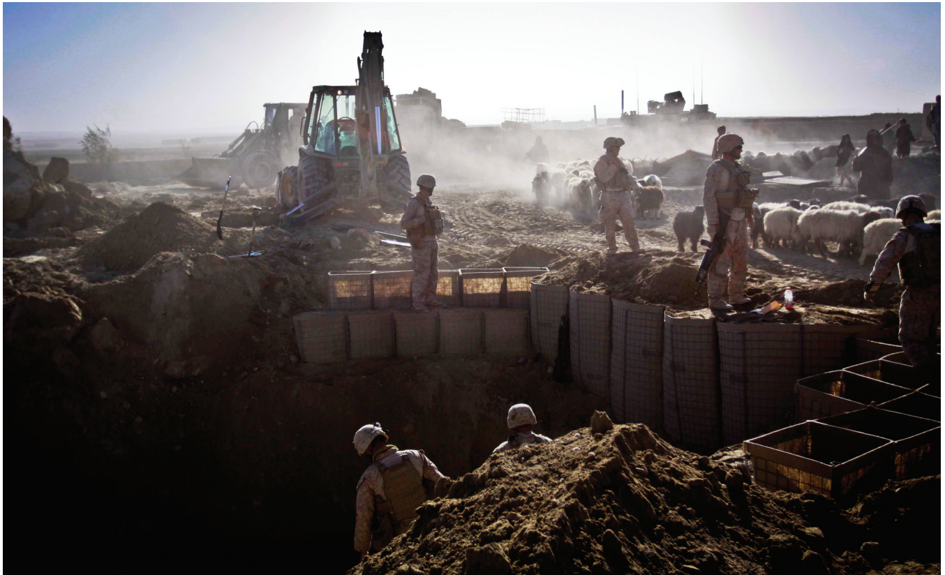
Marines building a bridge, Helmand province, Afghanistan (U.S. Marine Corps photo, December 2010).
