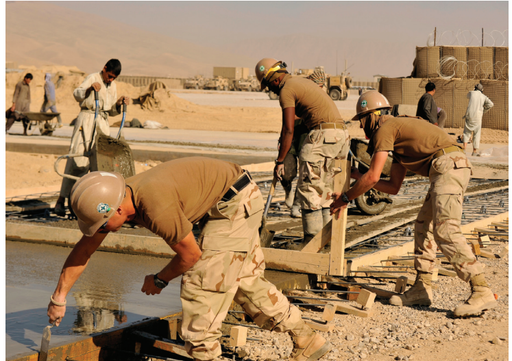
U.S. sailors and Afghan contractors building helicopter landing pads at base in Afghanistan (U.S. Navy Photo, Nov. 2010).
