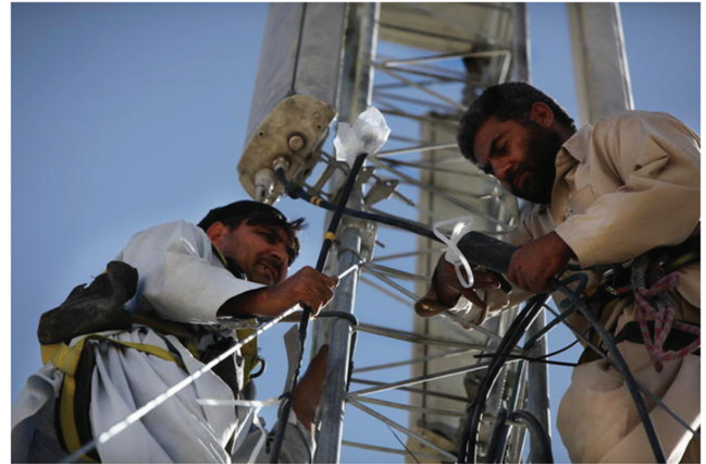
Afghan contractors working at new cellular telephone tower, Helmand province, Afghanistan (U.S. Marine Corps photo, Oct. 2010).
