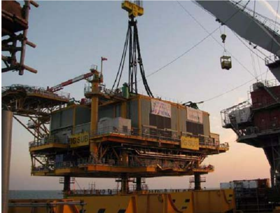
Figure 46: The Stanislav Yudin seen installing 2150 t Greater Gabbard substation off Harwich (Courtesy Adri Haasnoot-Piling Engineer Stanislav Yudin).
