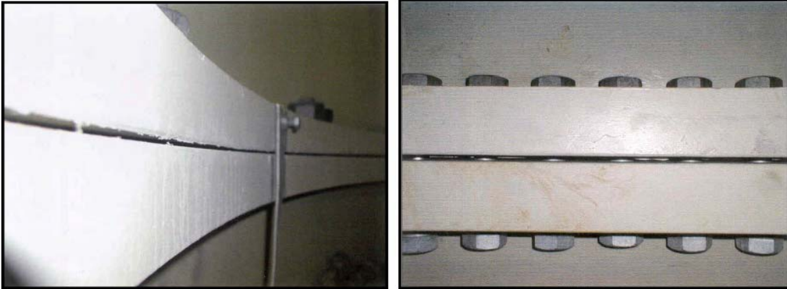
Fig. 2: Imperfect ring flange connections before pre-stressing
