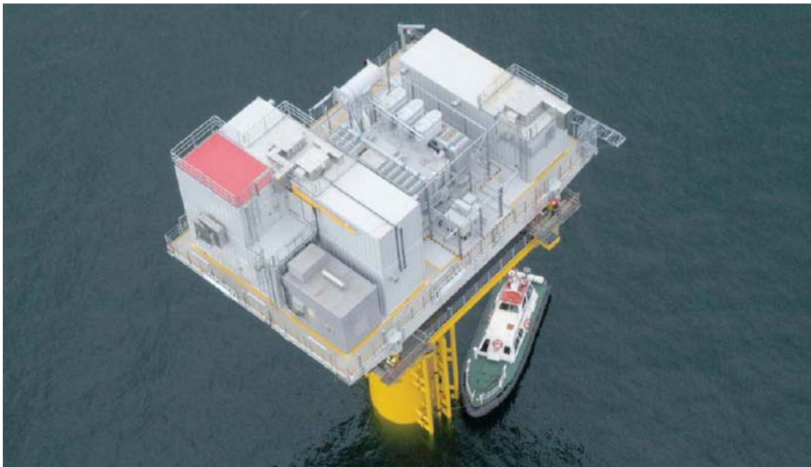
Figure 47: Areva HV/AC Transformer Substation: Barrow
