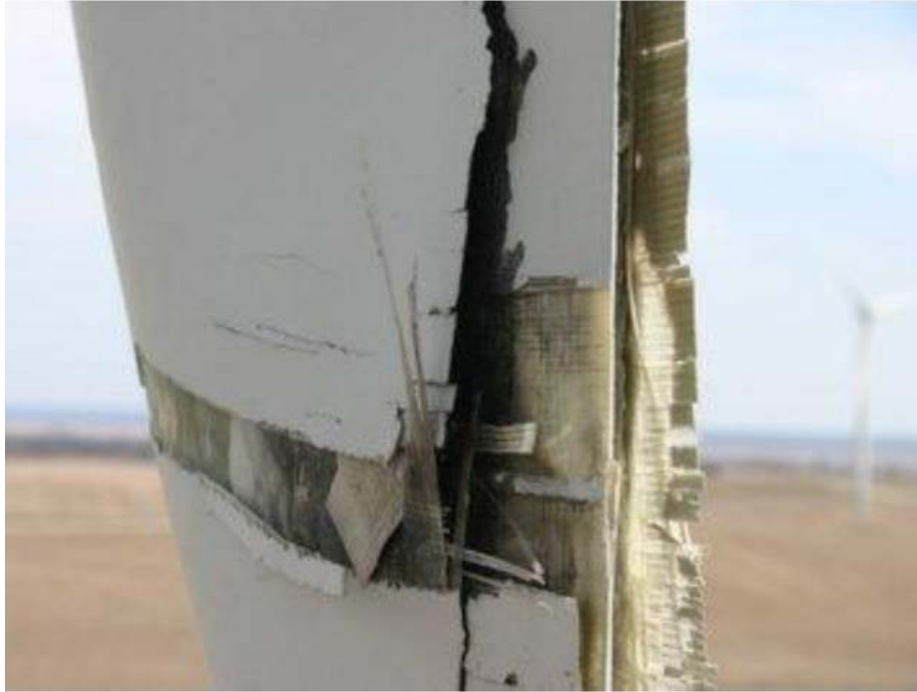
Figure 27: Example of Lightning Damage [Ref. 3.7.8].
