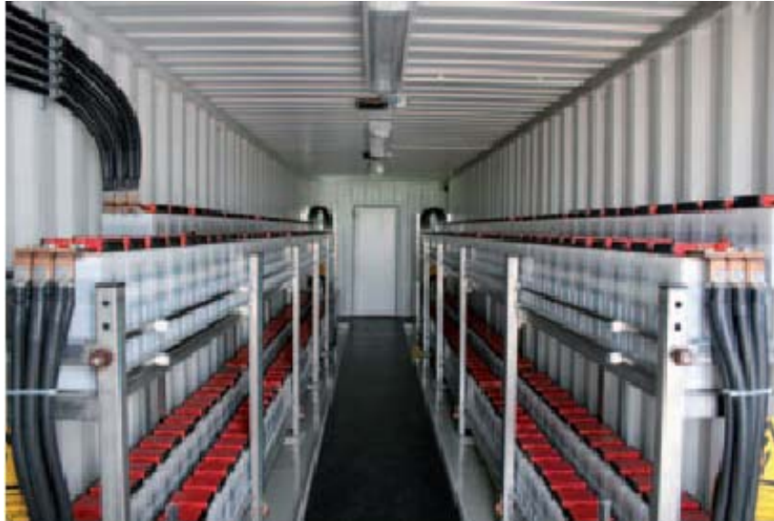
Figure 14: "The SAFT NiCd cells have a power capacity of 3000 kw for 2 minutes" Ref: Enercon Windblatt Magazine 03 2009.
