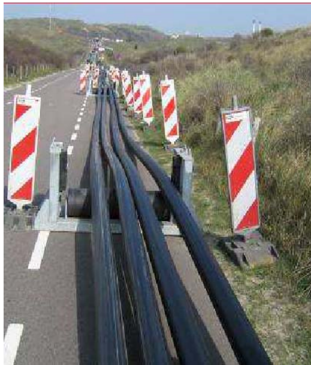
Figure 66: Cables on shore: Nuon offshore wind farm: [Ref. 7.9].
