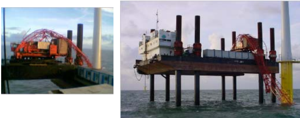
Figure 4. North Hoyle Crane Collapse
