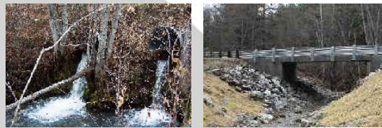
Little Browns Creek, Weaver Creek, Trinity River. A fish passage barrier 300 ft long culvert with 8-foot jump was replaced with a bridge. 2.5 miles of historic coho and steelhead habitat opened.
