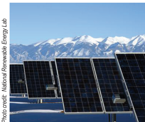
Solar panels, Alamosa Photovoltaic Plant
