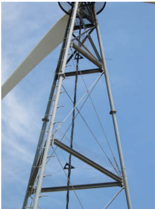
Photo 7-6. Mesh hardware cloth (“chicken wire”) used as perch guard on a lattice tower.
