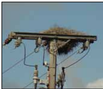
MONK PARAKEETS CAN DAMAGE POWER STRUCTURES WITH THEIR NESTS, FLORIDA POWER & LIGHT COMPANY
