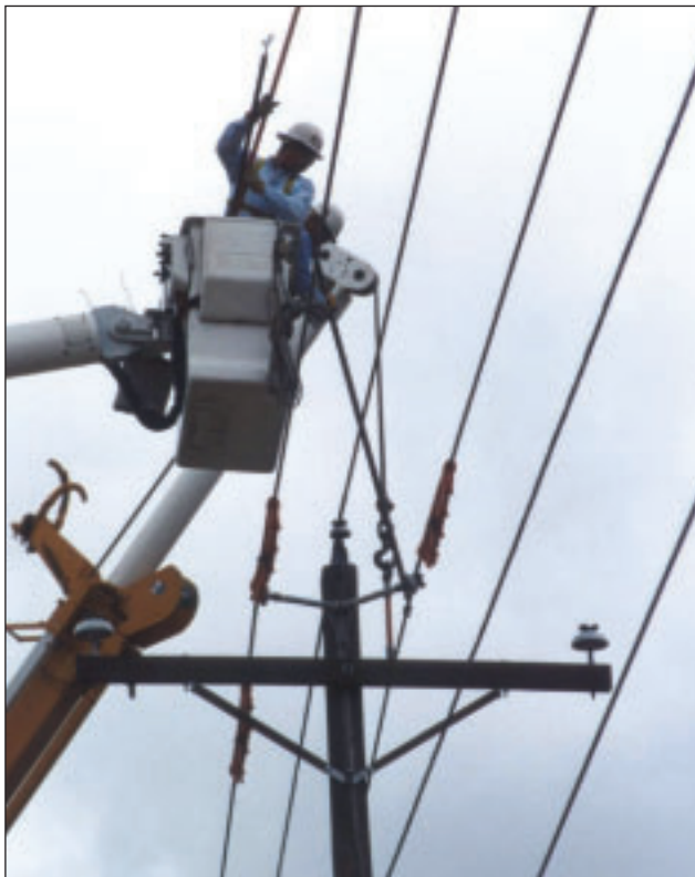
FIGURE 7.2: Reframing a crossarm to prevent avian electrocutions.
