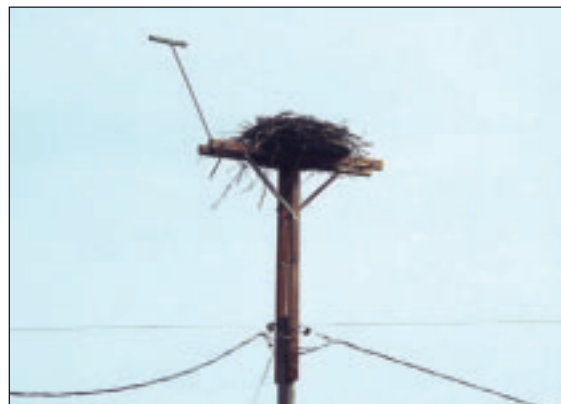
FIGURE 6.11: A nest platform built atop a pole using crossarms to extend the platform above the conductors. This design also includes an optional elevated perch to attract ospreys. The perch should be perpendicular to the prevailing wind.
