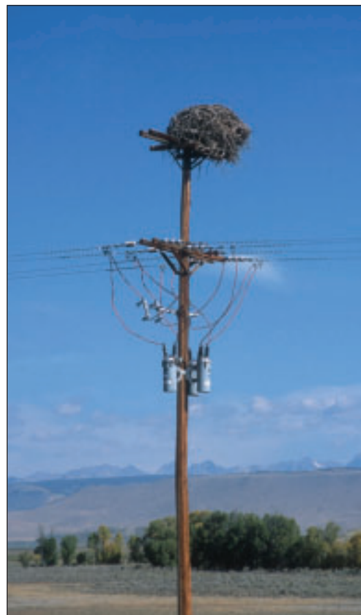
FIGURE 6.16: Osprey nest in Wyoming atop double dead-end pole. Nesting material that may drop onto the conductors or equipment poses fire, outage, and equipment damage risks.
