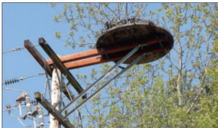
FIGURE 6.10: Osprey nest platform design developed by Portland General Electric. The platform is constructed from the end of a 1.5-meter (m) (5-foot [ft]) diameter wooden cable spool with coated cable along the edge to contain nest material. Utilities should ensure energized parts and equipment below the nest are covered to prevent electrocution of birds or outages from nest material. Consumer's Power, Inc. retrofitted this pole to their avian-safe standards.
