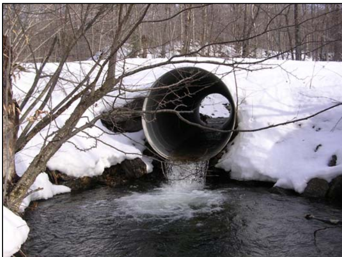
Culvert causing a passage barrier to brook trout in Stevensville Brook (Courtesy Chris Smith- USFWS)
