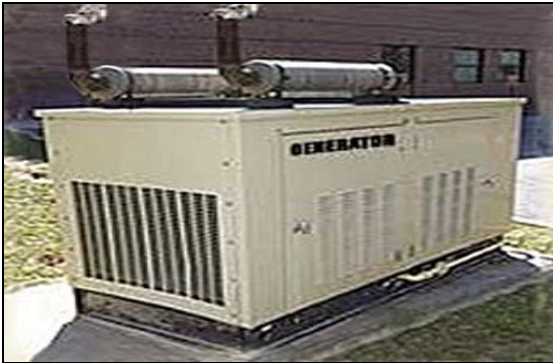
Back-up generator in case of power outage
