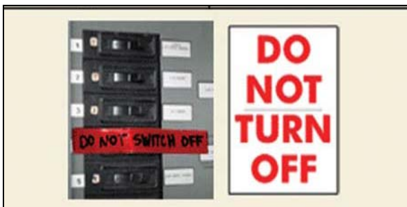
Label fuses/circuit breakers
