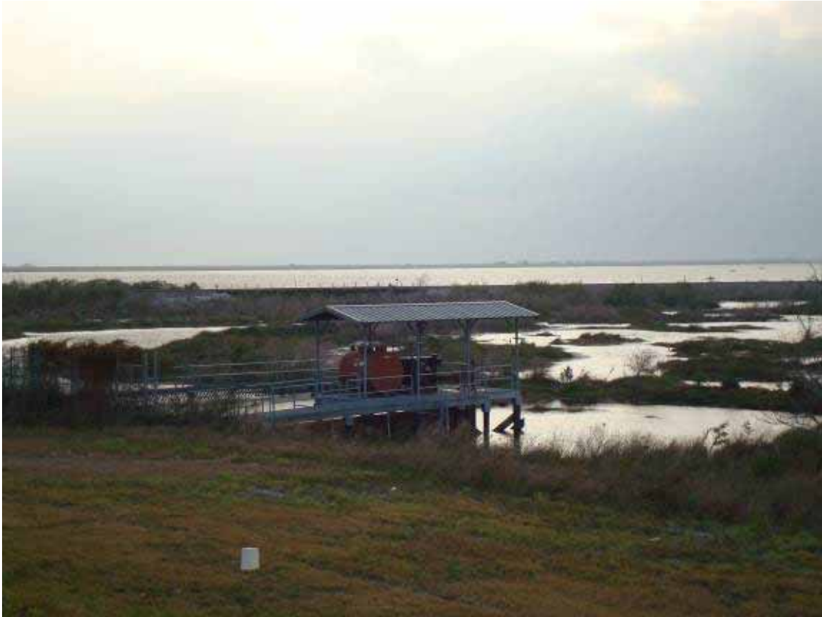
Photograph 4. Bayou Sauvage NWR Pump Station
