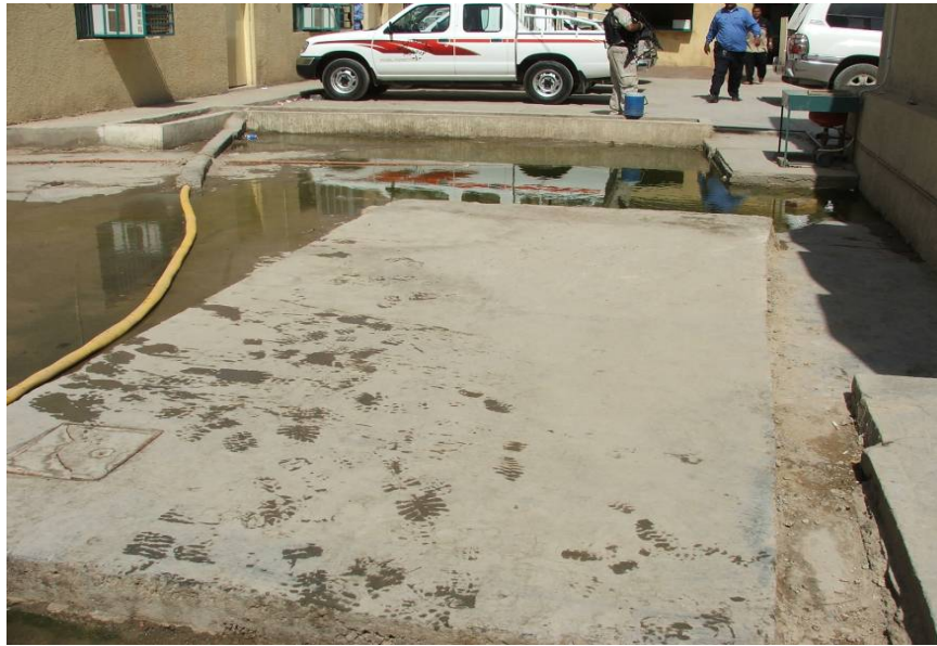
Site Photo 3. Septic Tank Cover with Un-drained Water
