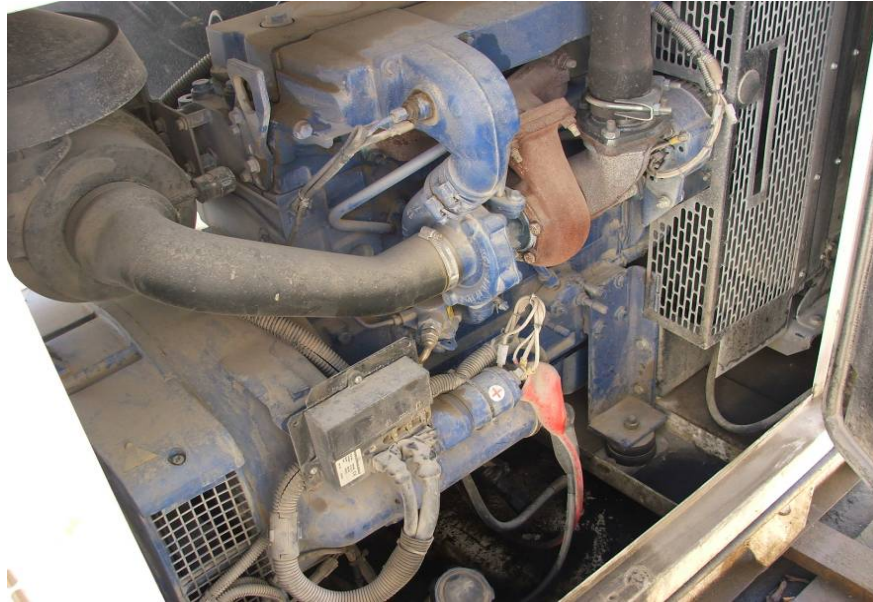
Site Photo 5. 82.5 kVA Generator
