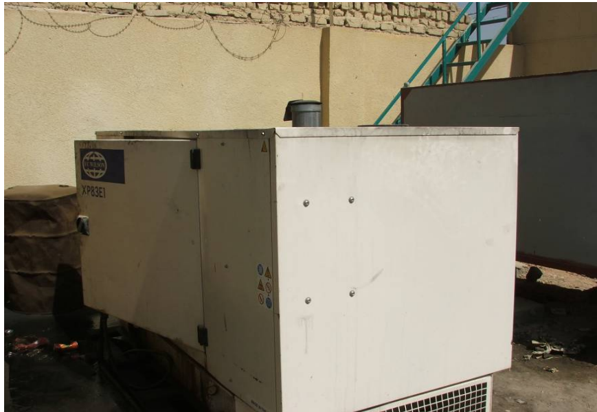
Site Photo 4. Generator Housing
