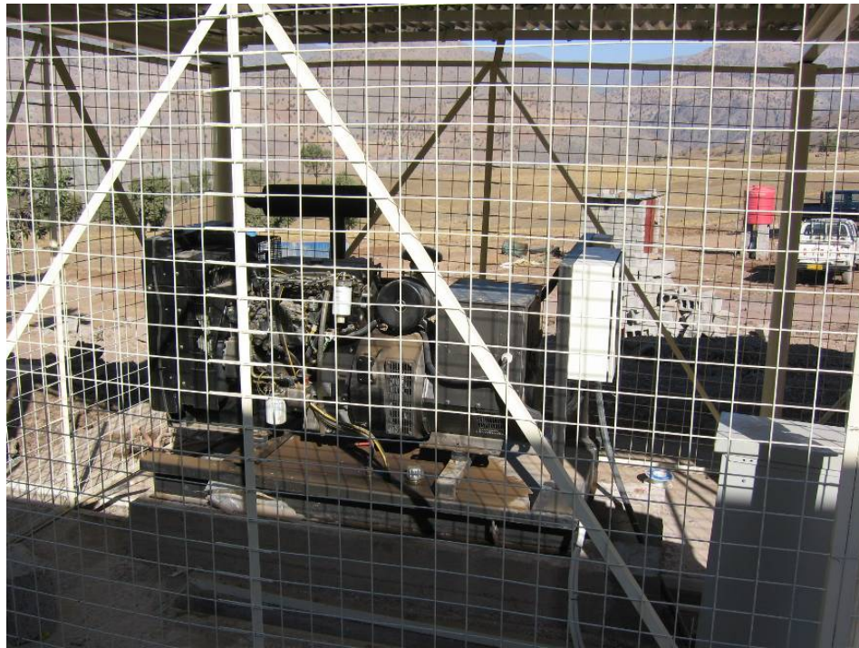
Site Photo 45. Generator Unit (Azmic #602 Border Post)
