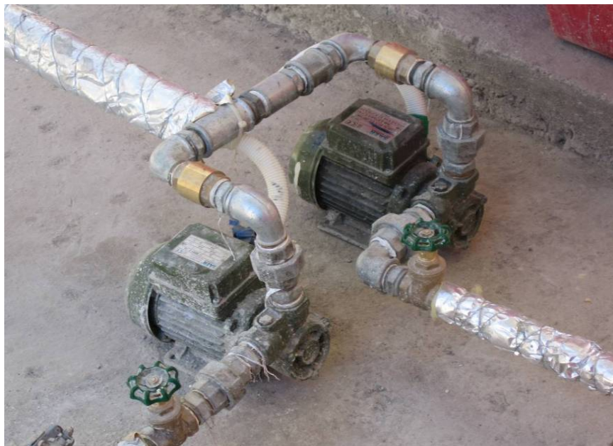
Site Photo 25. Two 1/2-Horsepower Pumps (Safrah #634 Border Post)
