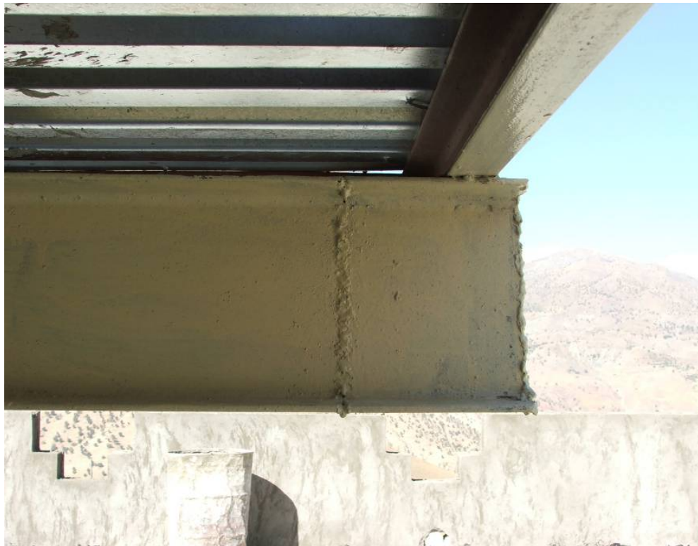
Site Photo 5. Lateral I-Beam Member – Cut Short and Welded (Issawa #604 Border Post)
