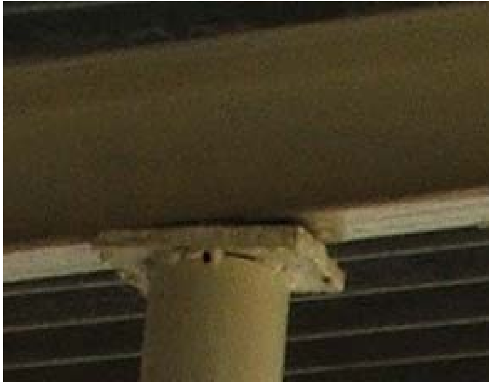
Site Photo 8. Upper Column Bearing Plate Showing Incomplete Welds (Safrah #634 Border Post)
