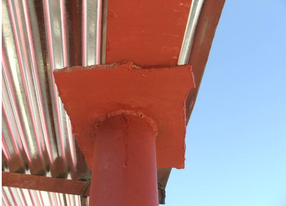
Site Photo 4. Bearing Plate on Roof-Mounted Water Tank Canopy (Azmick #602 Border Post)
