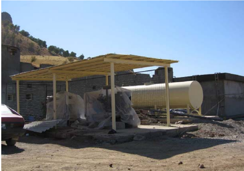
Site Photo 54. Two Generator Units and Fuel Tank (Issawa #604 Border Post)
