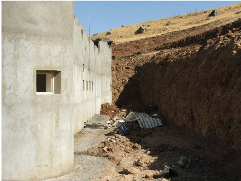
Site Photo 51. Right Exterior Wall (Issawa #604 Border Post)
