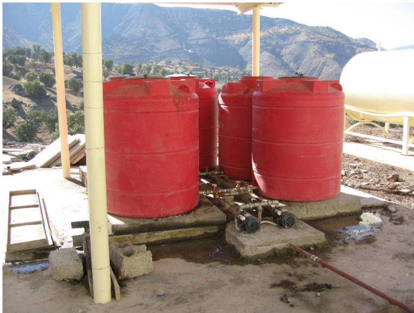
Site Photo 47. Ground-Mounted Storage Tanks, Pumps, and Piping (Azmic #602 Border Post)
