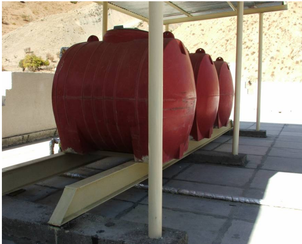
Site Photo 23. Three Roof Mounted Water Storage Tanks (Safrah #634 Border Post)
