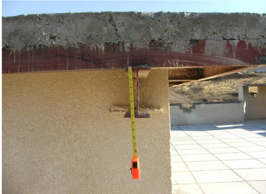
Site Photo 3. I-Beam Lateral Member Not Properly Aligned (Marwa #628 Border Post)
