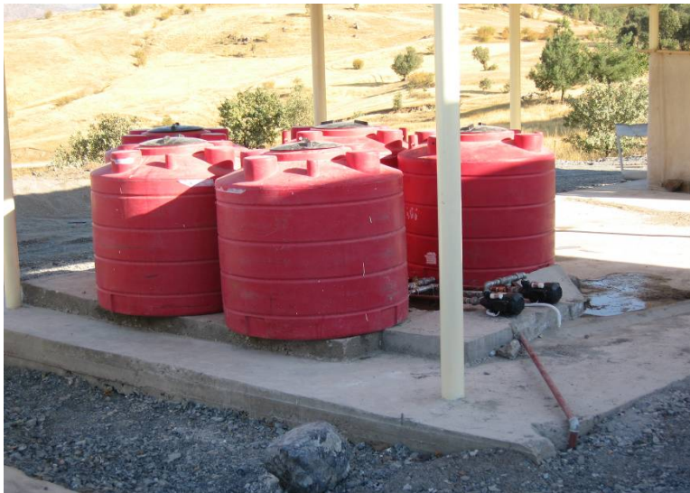
Site Photo 37. Ground-Mounted Water Storage Tanks (Marwa #628 Border Post)
