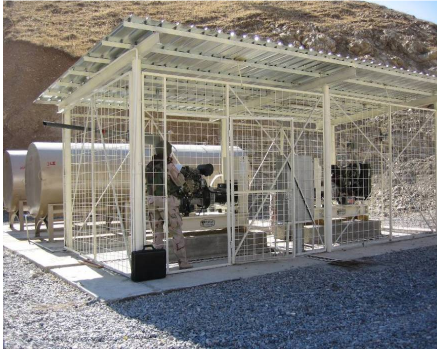
Site Photo 20. Two Generator Units, Metal Enclosures, and Fuel Tanks (Safrah #634 Border Post)
