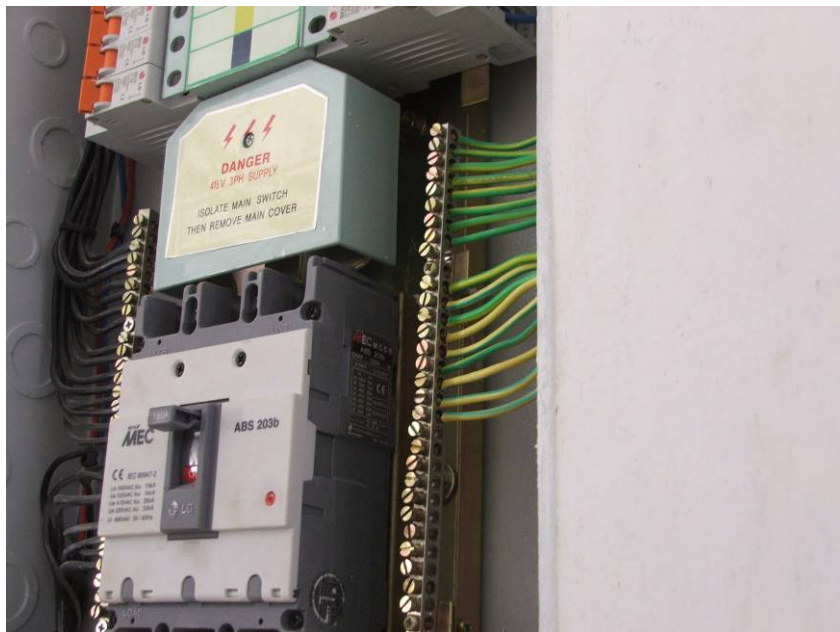
Site Photo 43. Electrical Circuit Breaker Panel (Azmic #602 Border Post)
