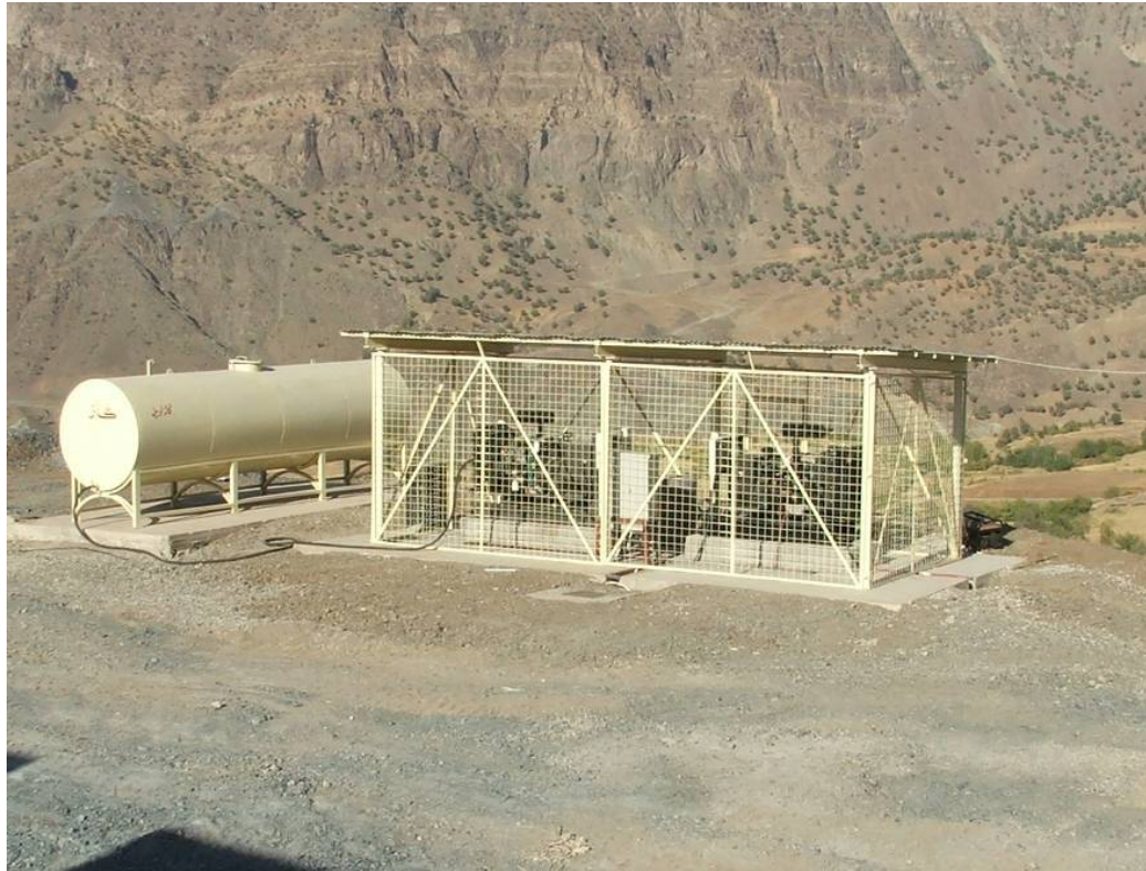
Site Photo 35. Generator and Fuel Tank (Marwa #628 Border Post)
