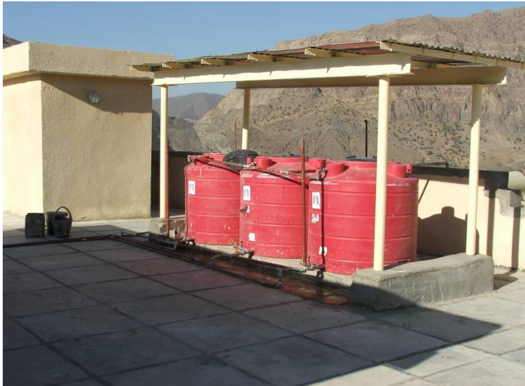
Site Photo 36. Roof-Mounted Water Storage Tanks (Marwa #628 Border Post)
