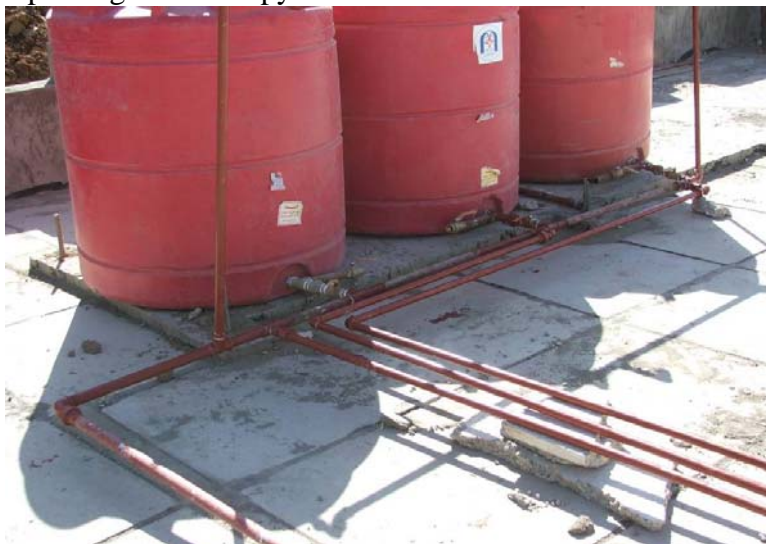
Site Photo 55. Roof-Mounted Water Tanks (Issawa #604 Border Post)
