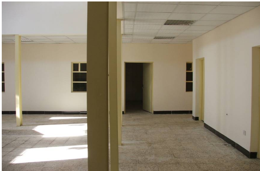
Site Photo 1. Steel I-Beam Columns – Not Plumb (Marwa #628 Border Post)
