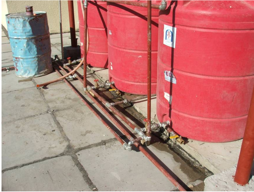
Site Photo 46. Roof-Mounted Water Storage Tanks and Piping (Azmic #602 Border Post)
