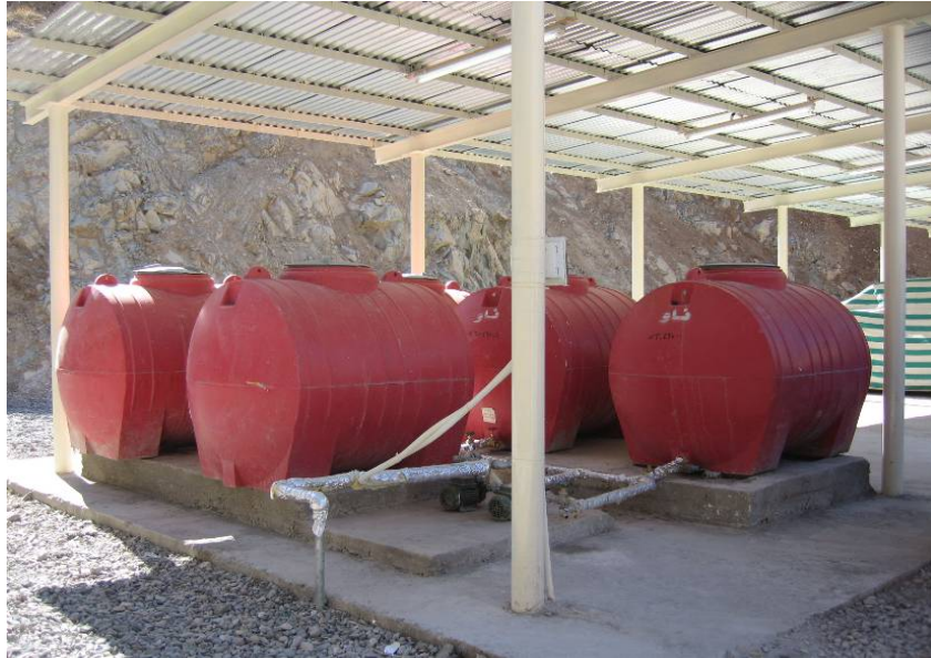
Site Photo 24. Five Ground-Mounted Water Storage Tanks (Safrah #634 Border Post)
