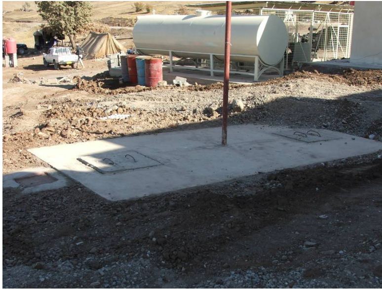
Site Photo 48. Septic Tank and Access Ports (Azmick #602 Border Post)
