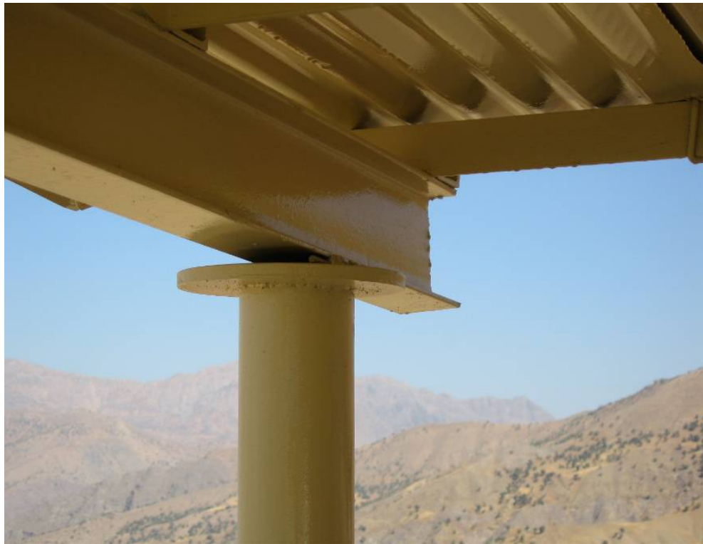
Site Photo 9. Upper Column Bearing Plate Only Connected On One Edge (Issawa #604 Border Post)
