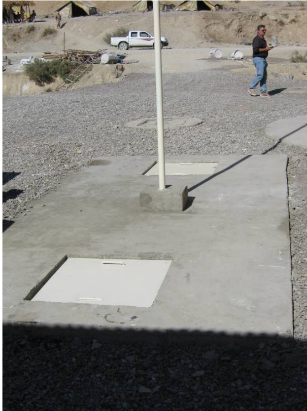
Site Photo 26. Septic Tank (Safrah #634 Border Post)
