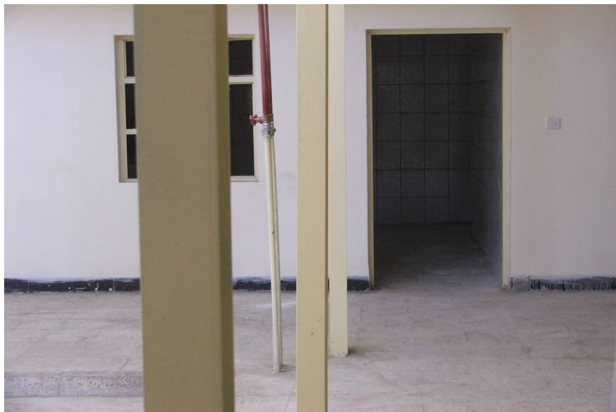
Site Photo 2. Steel I-Beam Columns – Not Plumb (Issawa #604 Border Post)
