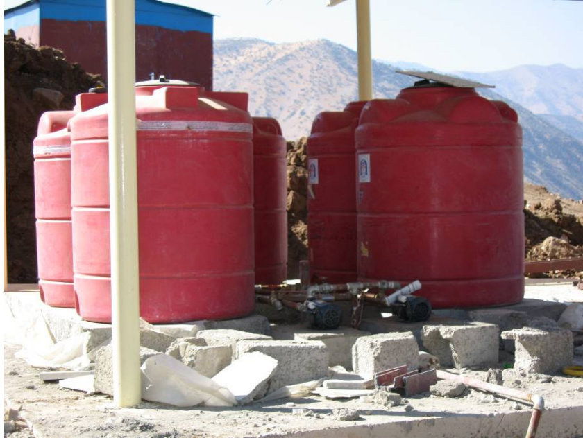
Site Photo 56. Ground Mounted Water Tanks (Issawa #604 Border Post)
