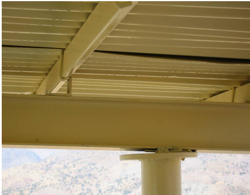
Site Photo 10. Upper Column Bearing Plate Only Connected On One Edge (Issawa #604 Border Post)
