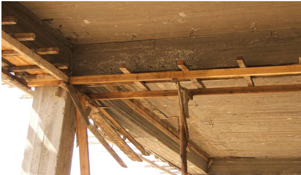
Site Photo 5. First Floor Ceiling Concrete Beam with Concrete Segregation
