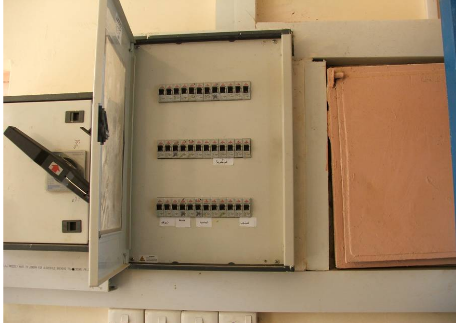
Site Photo 6. Circuit Breaker Panel
