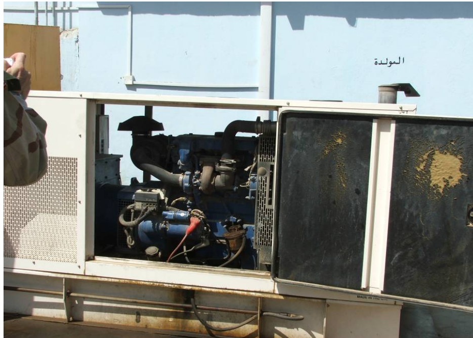
Site Photo 8. 82.5 kVA Generator
