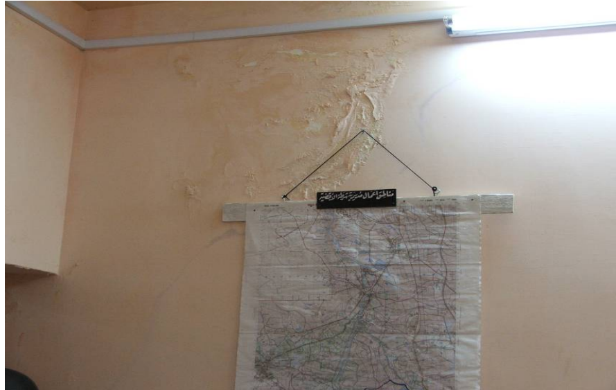
Site Photo 3. Damaged Interior Room Wall
