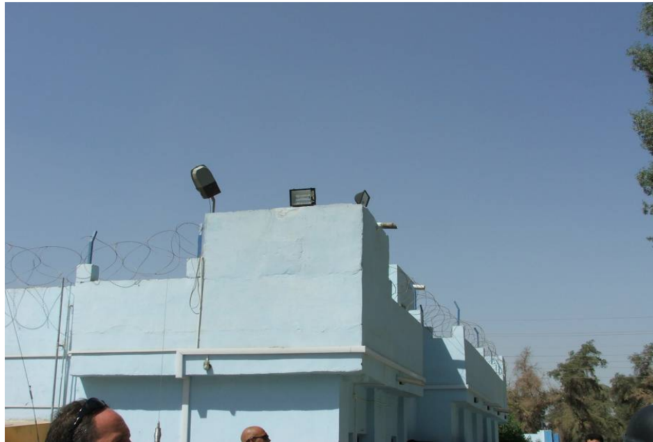
Site Photo 7. Exterior Mounted Lights on Police Station Walls
