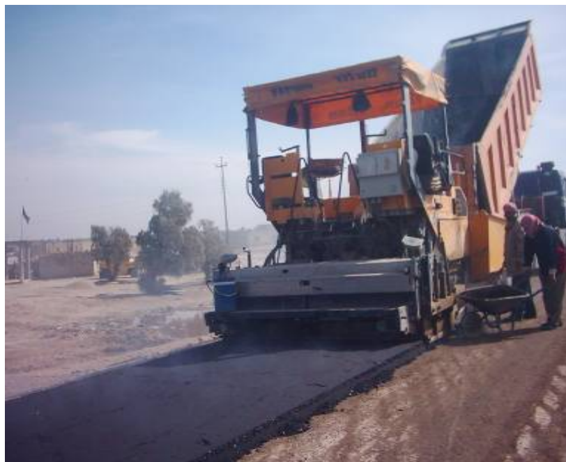
Site Photo 5. Placing and spreading asphalt concrete pavement –Photo provided by USACE
