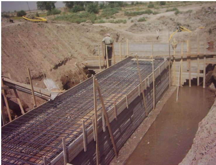
Site Photo 11. Construction of reinforced concrete box culvert – Photo provided by USACE.
