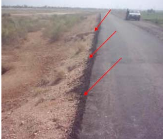
Site Photo 9. Asphalt mix sloughing off along pavement edge due to poor sub-base and fill construction – Photo provided by USACE
