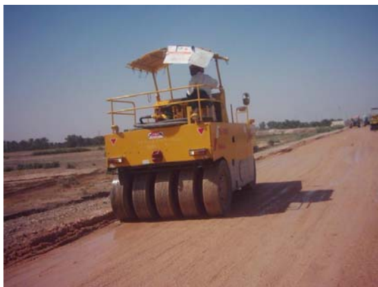
Site Photo 3. Compacting the sub-base with a pneumatic rubber tired roller – Photo provided by USACE
