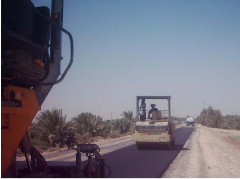
Site Photo 6. Steel wheel roller behind paver compacting the asphalt concrete layer – Photo provided by USACE
