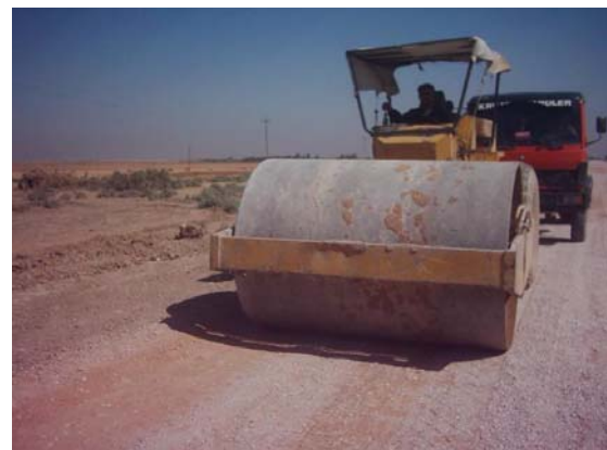
Site Photo 4. Compacting the sub-base with a steel wheeled roller – Photo provided by USACE
