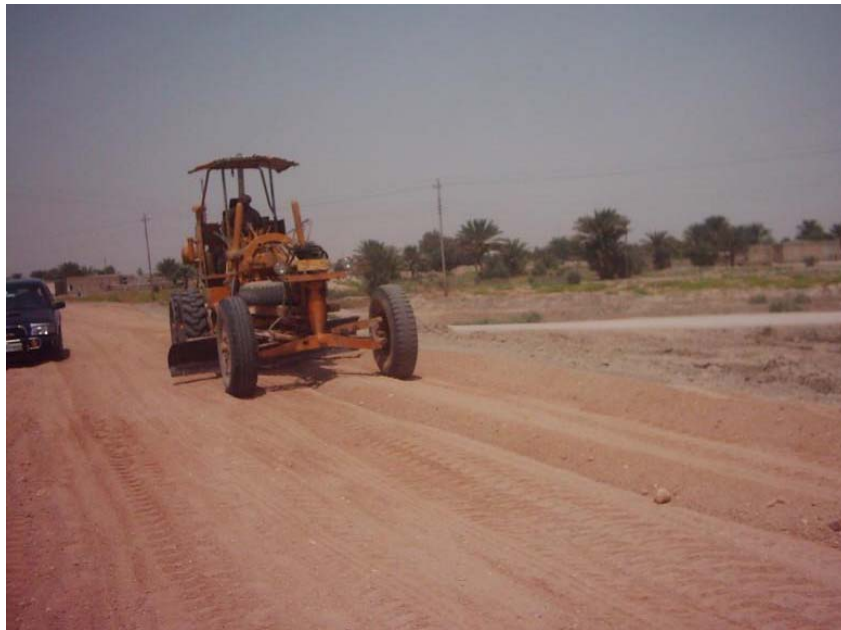
Site Photo 1. Contractor motor grader leveling the sub-base – Photo provided by USACE
