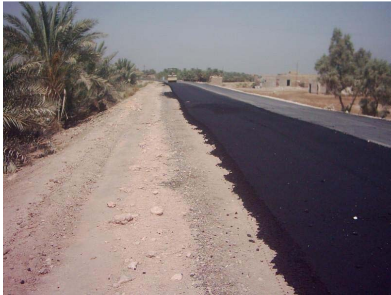
Site Photo 8 – Asphalt along edge that is “Sloughing Off of the Mat” – Photo provided by USACE
