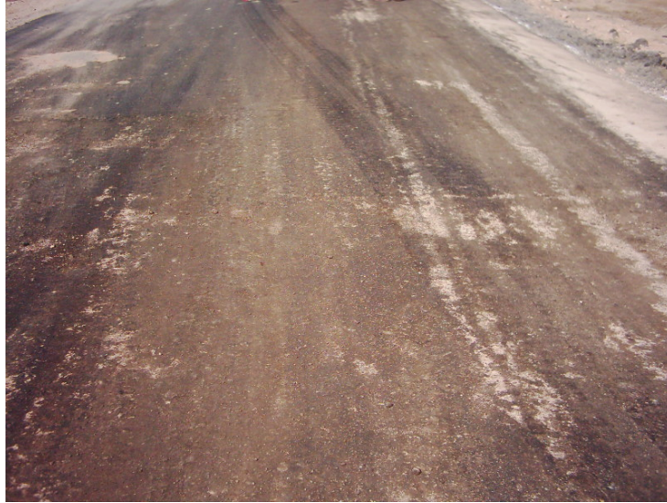
Site Photo 7. Lack of sufficient prime coat on sub-base prior to paving – Photo provided by USACE
