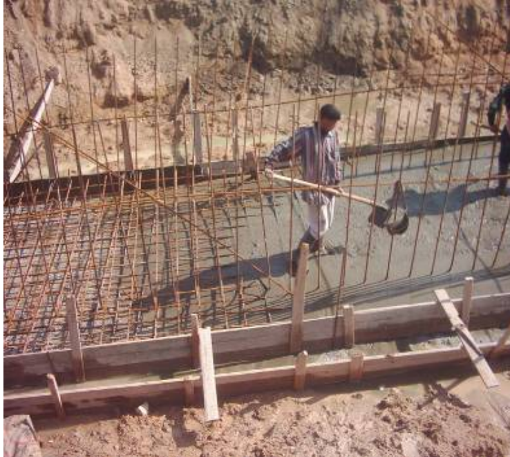
Site Photo 10. Construction of reinforced concrete box culvert foundation – Photo provided by USACE.
