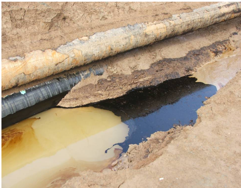
Site Photo 5. SIGIR Site Photo from February 2006. Oil leakage from existing pipeline
