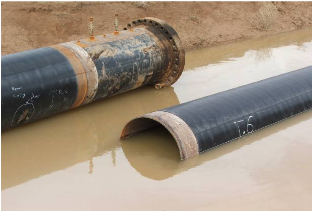
Site Photo 4. SIGIR Site Photo from February 2006. Additional pipe welding and repair work required
