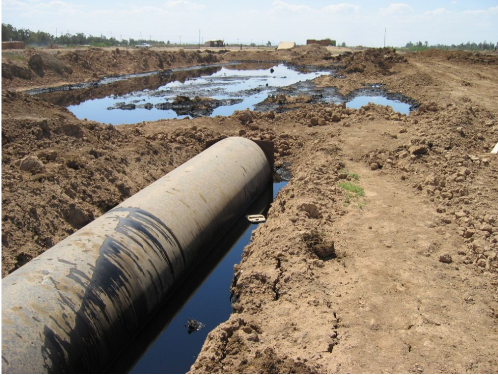
Site Photo 16. Pipe and oil near Riyadh Canal Crossing (Courtesy of PIJV – March 05)
