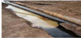
Site Photo 1. Example of Severe Corrosion of Existing Pipeline and Oil Leakage Task Force - Restore Iraqi Oil The U.S. Army Corps of Engineers (USACE) was assigned the responsibility to repair and upgrade the oil and gas pipelines in the Department of Defense's (DoD) northern Iraq Oil Field. The task force was established in 2003 as part of the Iraq Reconstruction Program (IRP). The task force was assigned prior to the beginning of Operations Enduring Freedom. The task force included the following:
