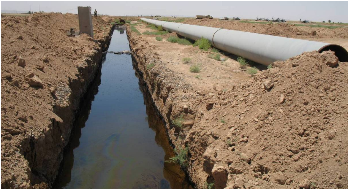
Site Photo 14. Welded pipe string and excavation at Zegeton Canal (Courtesy of IRMO - May 06)
