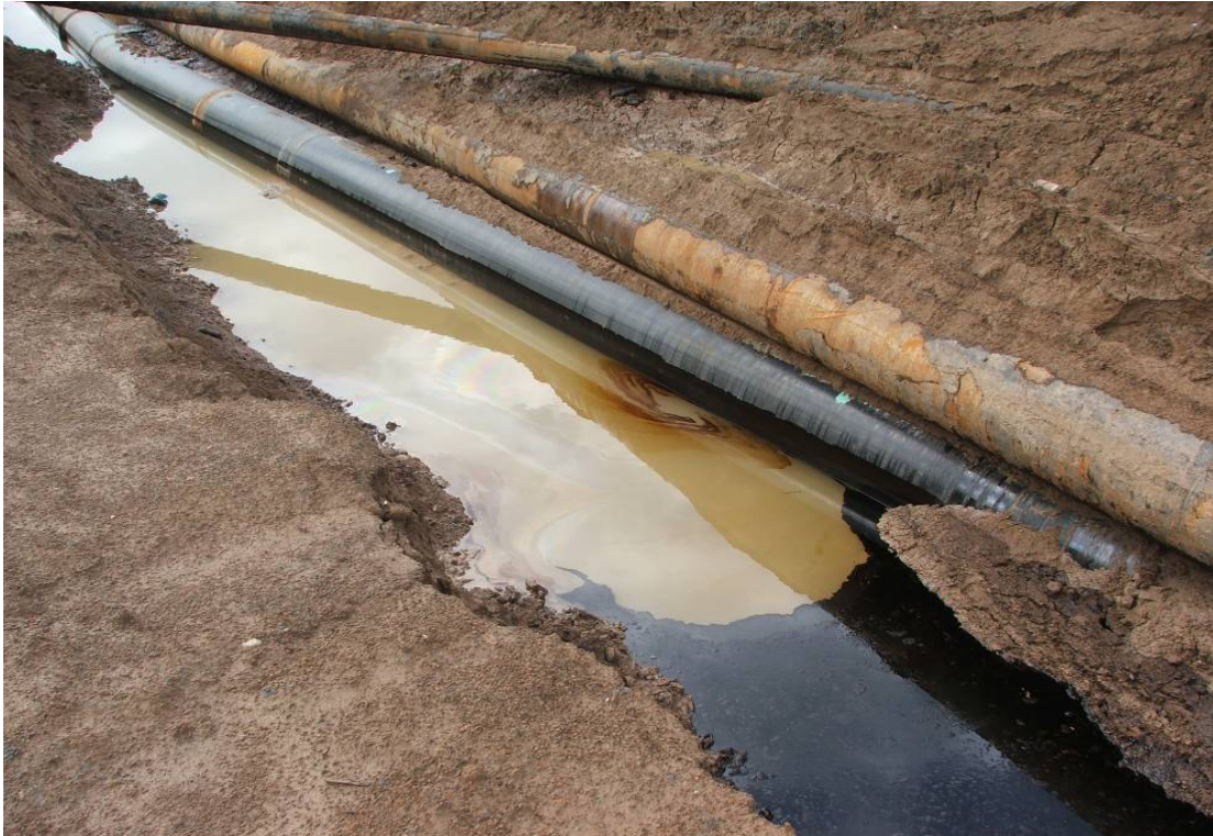
Site Photo 1. Example of severe external oxidation of existing pipeline and oil leakage
