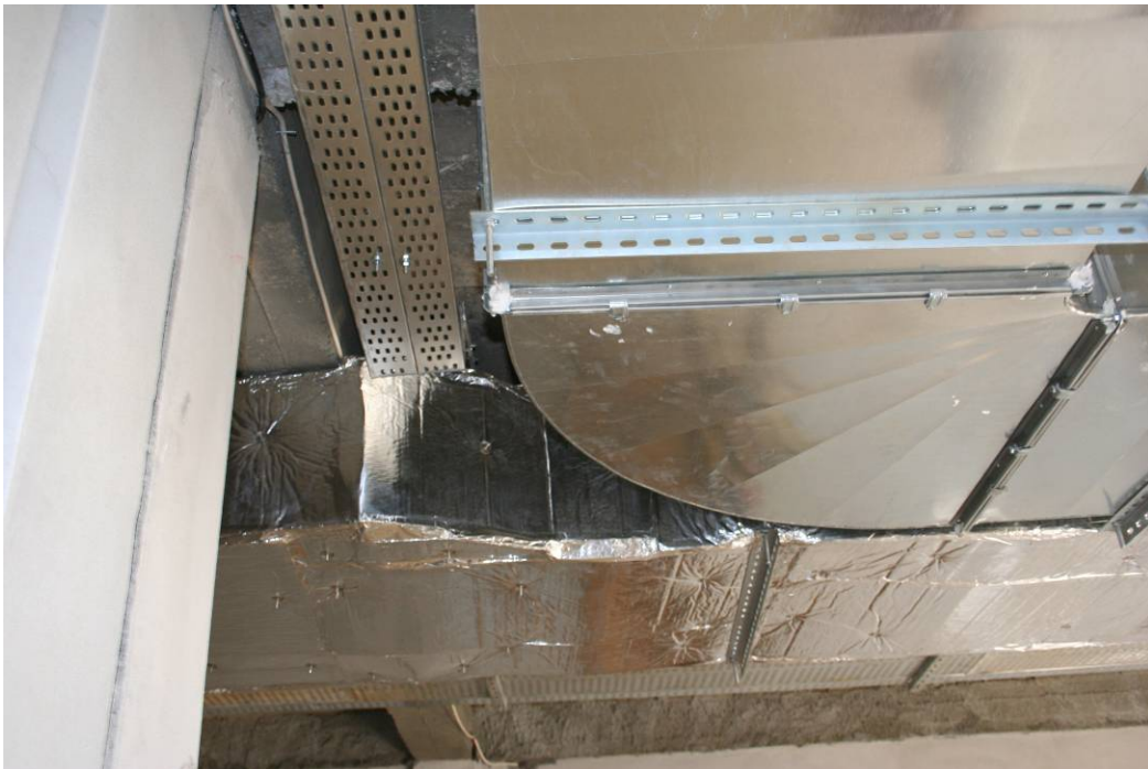
Site Photo 17. Cable tray and duct work were neatly installed in a confined area.
