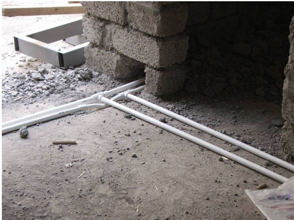
Site Photo 20. PVC pipe run along the floor was pressure tested before installation of floor tile.
