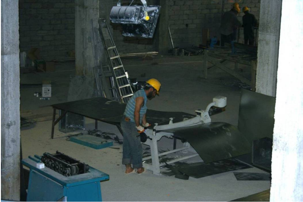
Site Photo 15. Centralized sheet metal shop was used to pre-fabricate ducts and other metal assemblies.
