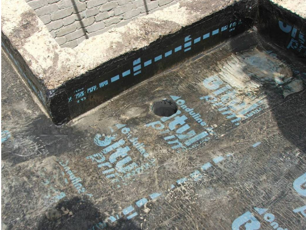
Site Photo 23. Topside view of rainwater collection basin with drain piping.
