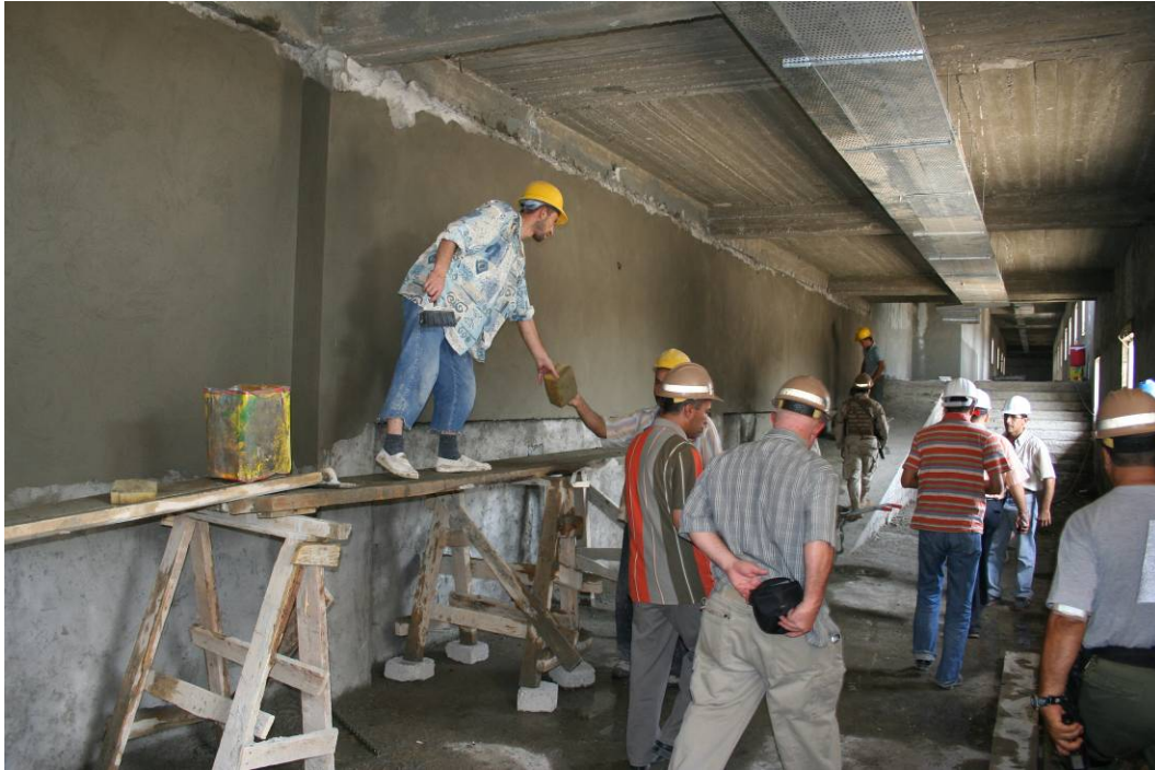
Site Photo 10. Workers finish an interior wall with a thin layer of concrete (plaster).
