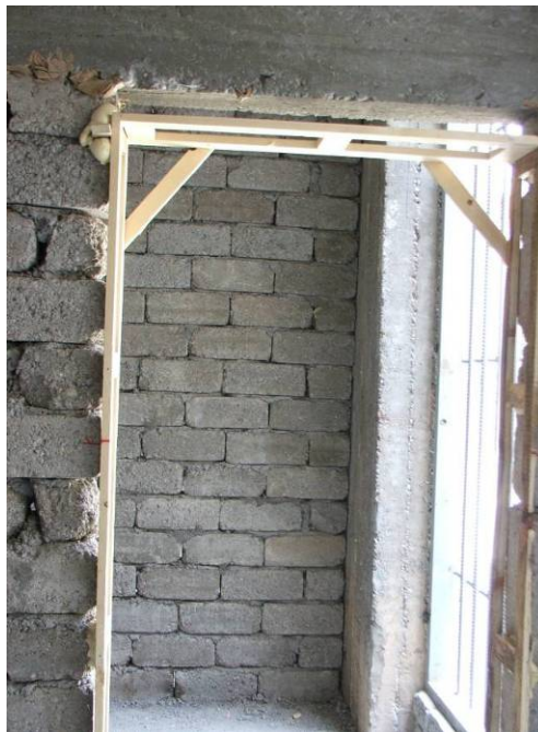
Site Photo 14. “Roughed-in” wooden doorway frame was positioned before finishing CMU wall.
