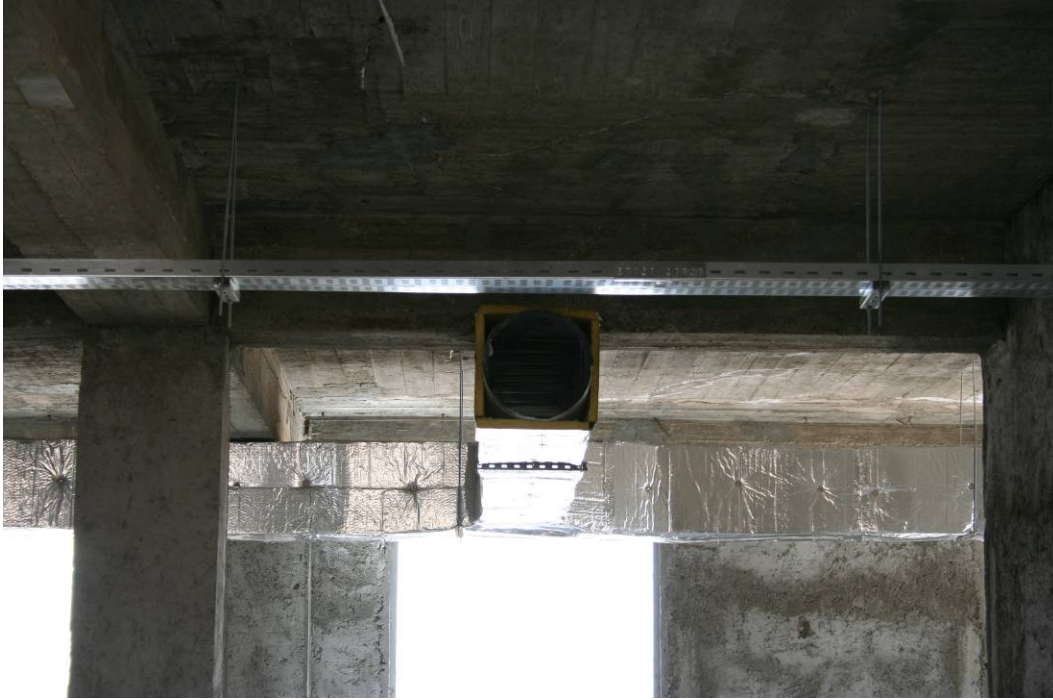
Site Photo 16. Ducts and cable trays throughout the facility appeared professionally installed.
