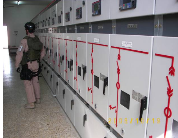
Site Photo 5. Al Hamdan substation distribution 11 kV switchgear panels at the time of the second assessment
