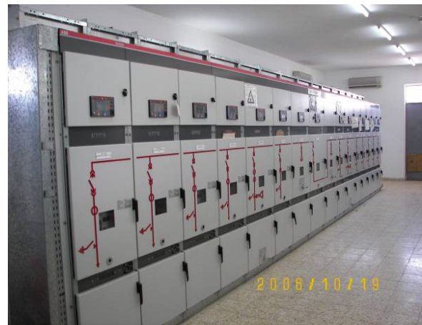
Site Photo 7. Al Seraji substation distribution 11 kV switchgear panels at the time of the second assessment
