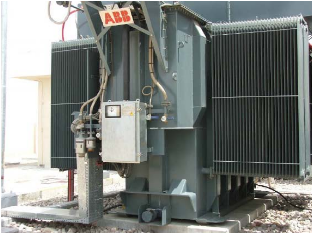
Site Photo 8. Al Hamdan 33/11 kV transformer at the first assessment
