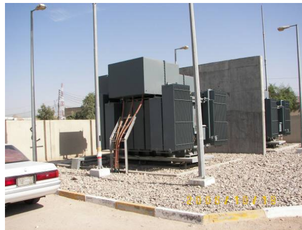
Site Photo 11. Al Seraji 33/11kV transformer at the second assessment
