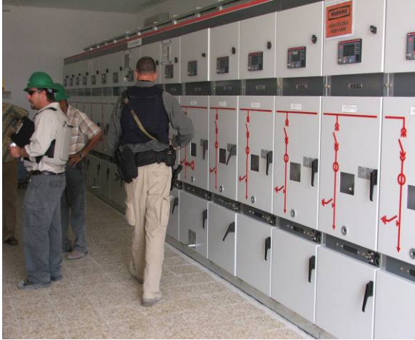
Site Photo4. Al Hamdan substation distribution 11 kV switchgear panels at the time of the initial assessment
