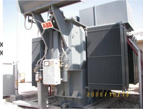
Site Photo 9. Al Hamdan 33/11kV transformer at the second assessment
