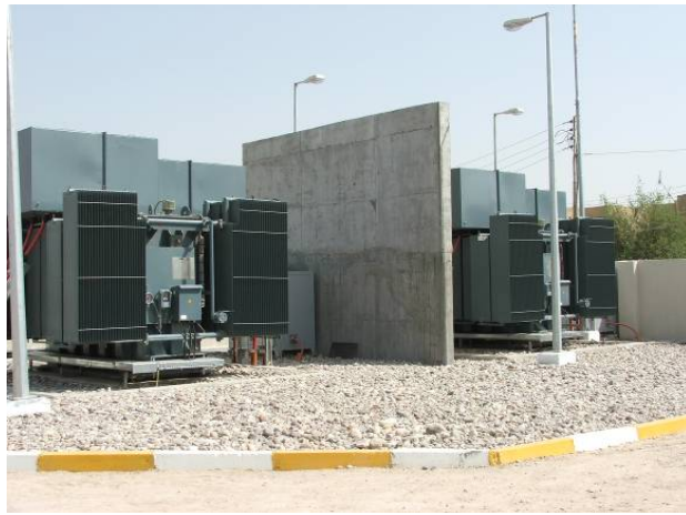
Site Photo 10. Al Seraji 33/11 kV transformer at the first assessment
