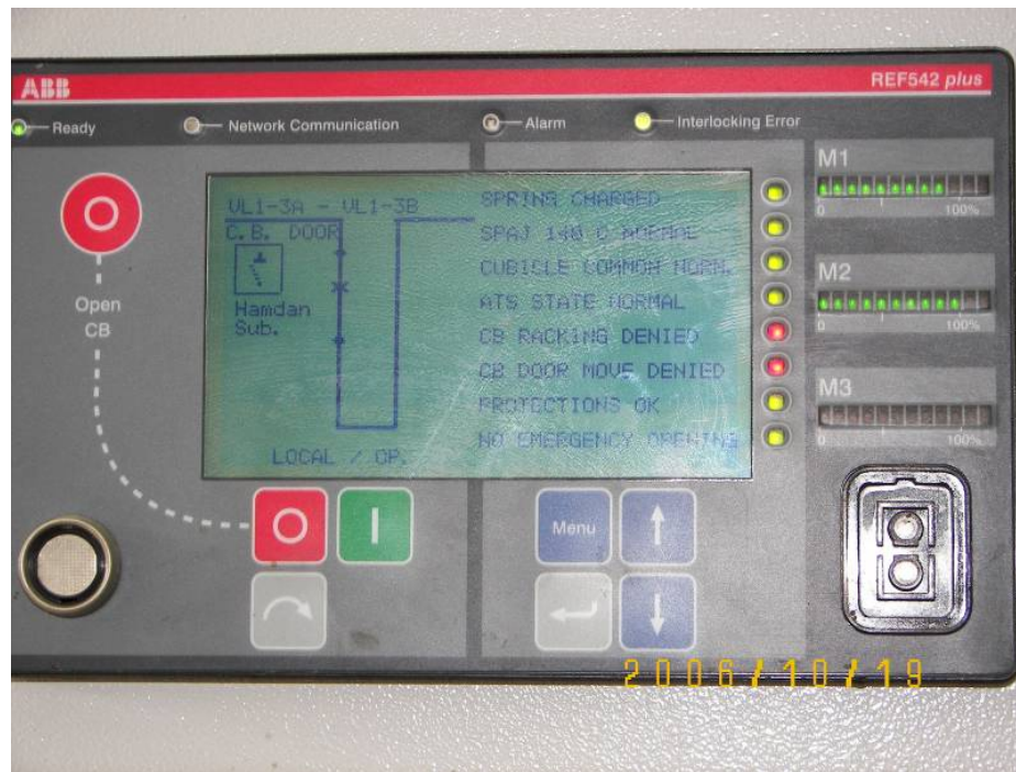
Site Photo 1. Switch panel display illustrating the closed distribution circuit
