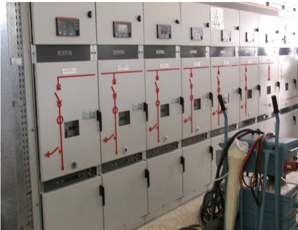
Site Photo 6. Al Seraji substation distribution 11 kV switchgear panels at the time of the initial assessment
