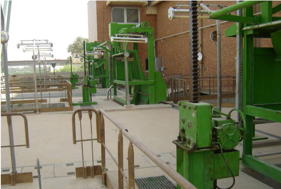
Site Photo 2. Sadr City Al Qana'at RWPS
