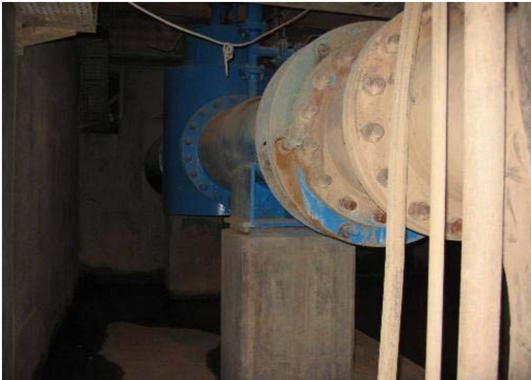
Site Photo 3. Sadr City Al Qana'at RWPS piping
