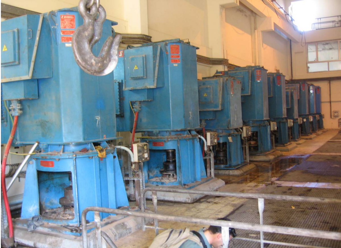
Site Photo 4. Vertical turbine pumps.
