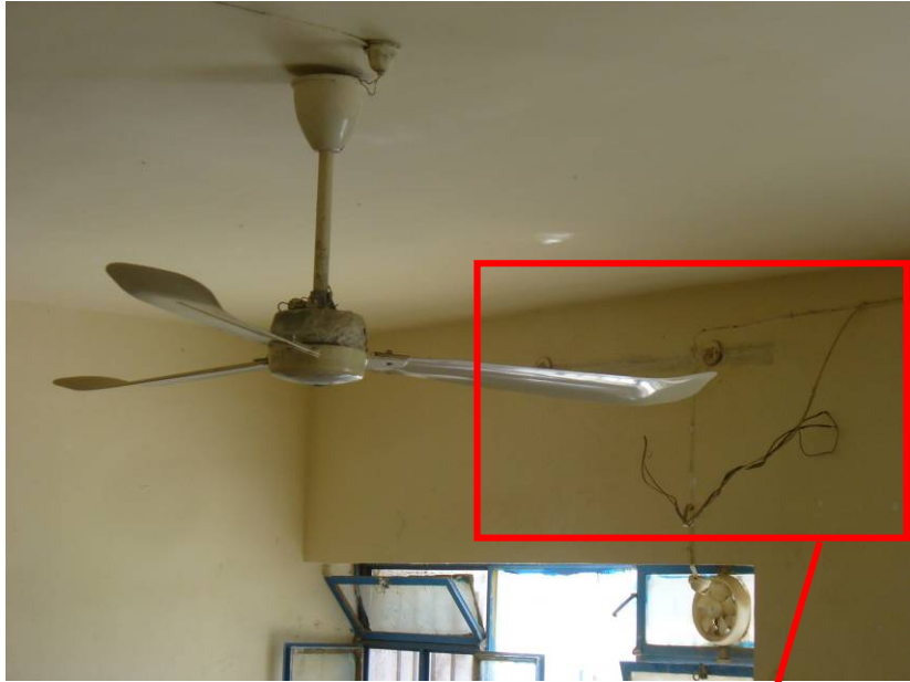
Site Photo 2. Loose electrical wiring before renovation (Photo courtesy of USACE)
