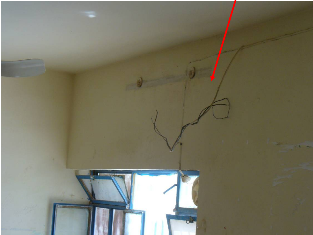
Site Photo 3. Broken light fixture with unsafe wiring before renovation (Photo courtesy of USACE)
