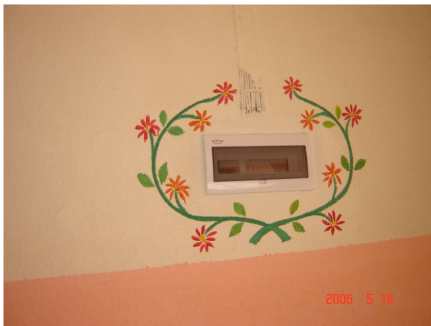
Site Photo 7. Interior painting and electrical rewiring after renovation (Photo courtesy of USACE)
