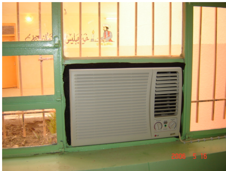
Site Photo 9. Proper air conditioning installation after renovation (Photo courtesy of USACE)
