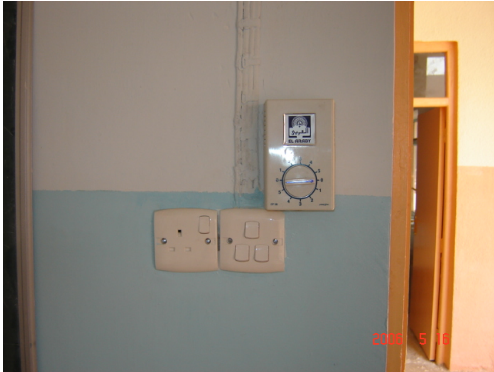
Site Photo 8. Correctly installed electrical switches and ceiling fan control after renovation (Photo courtesy of USACE)
