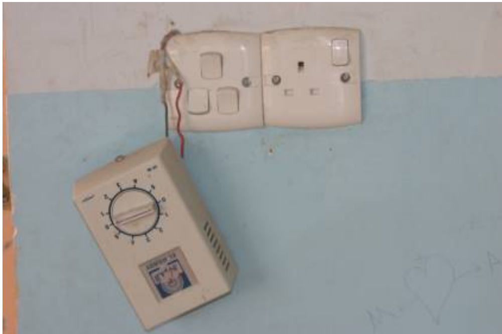
Site Photo 14. Tampered with wiring and added ceiling fan control after occupancy and use (Photo courtesy of USACE)
