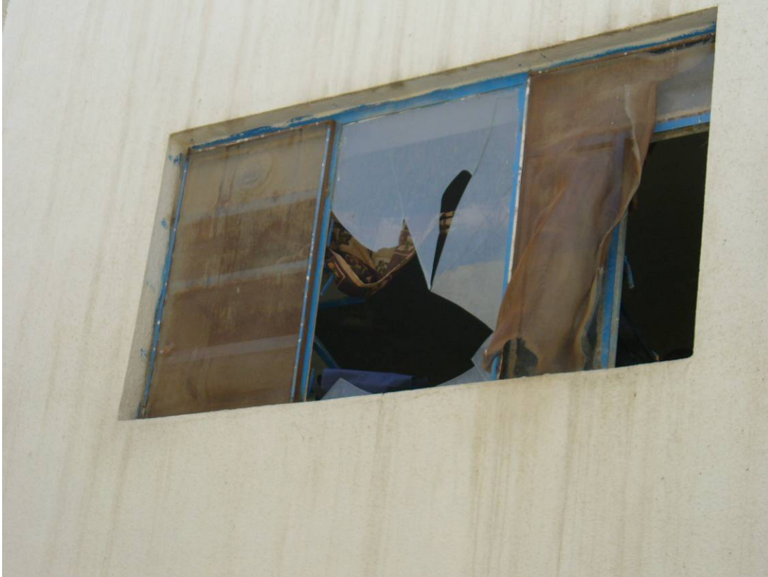
Site Photo 4. Safety hazard – broken windows at the school before renovation (Photo courtesy of USACE)
