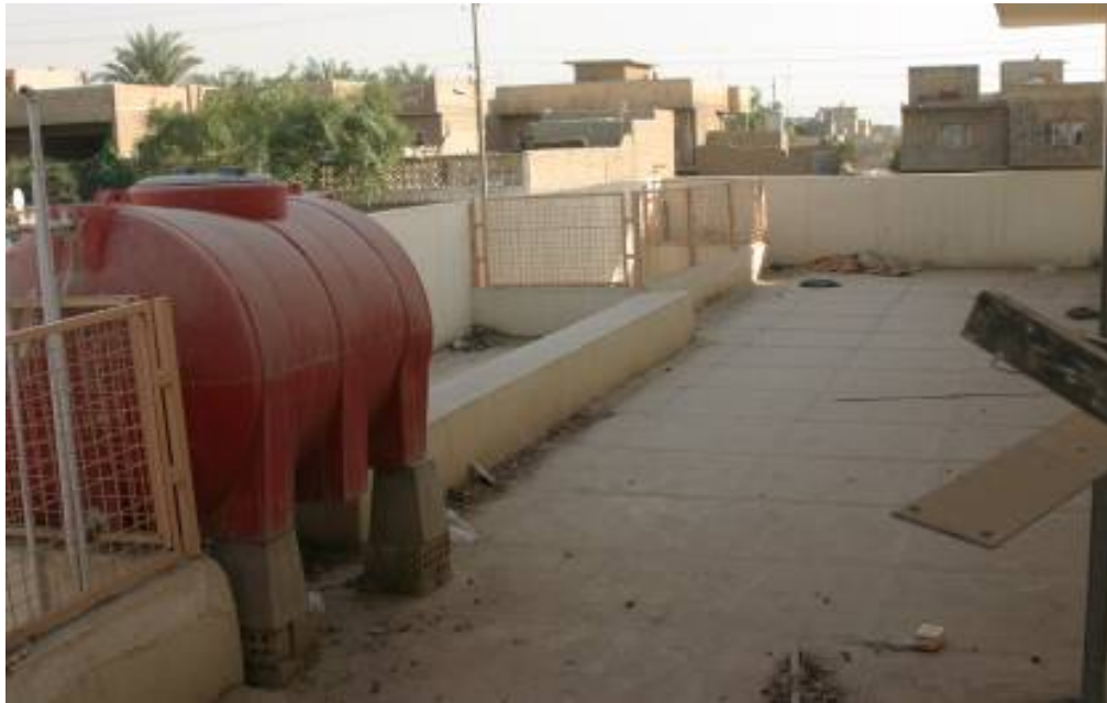
Site Photo 11. Roof maintenance after occupancy and use (Photo courtesy of USACE)
