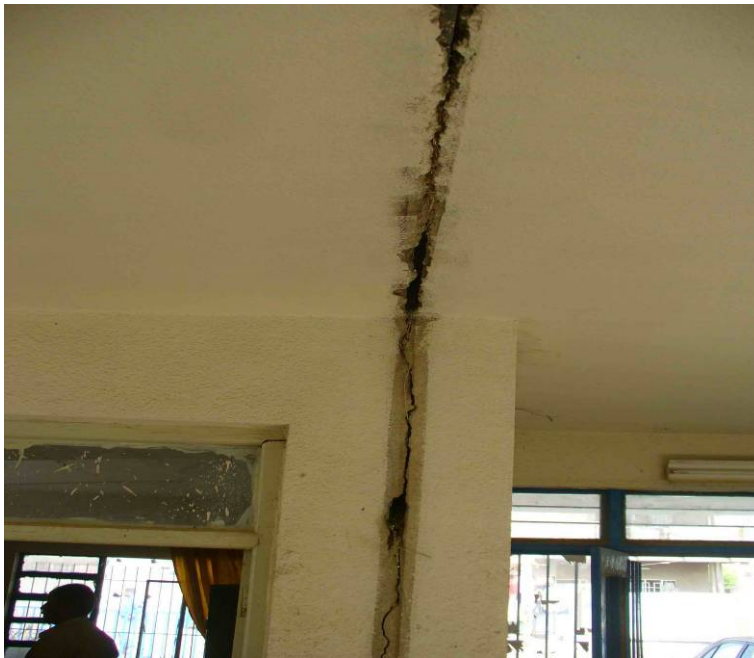
Site Photo 1. Open expansion joint before renovation (Photo courtesy of USACE)
