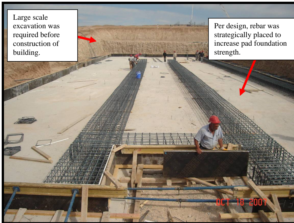
Site Photo 4. In single-story pad foundations, horizontal rebar assemblies designed to increase foundation strength were placed below the location of planned load bearing walls. (Photo courtesy of USACE)
