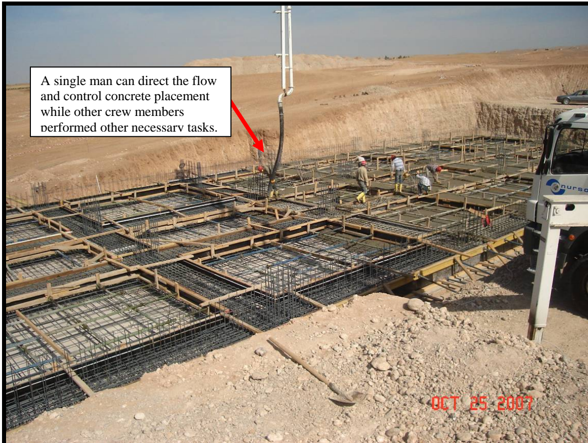
Site Photo 18. Concrete pump extension boom used to place concrete was handled by one man. (Photo provided by USACE)
