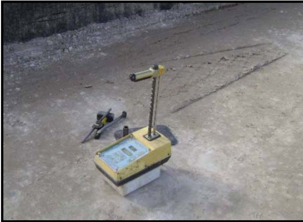
Site Photo 3. The contractor used modern equipment to perform compaction tests during the process fill and compact in layers. (Contractor provided photo)
