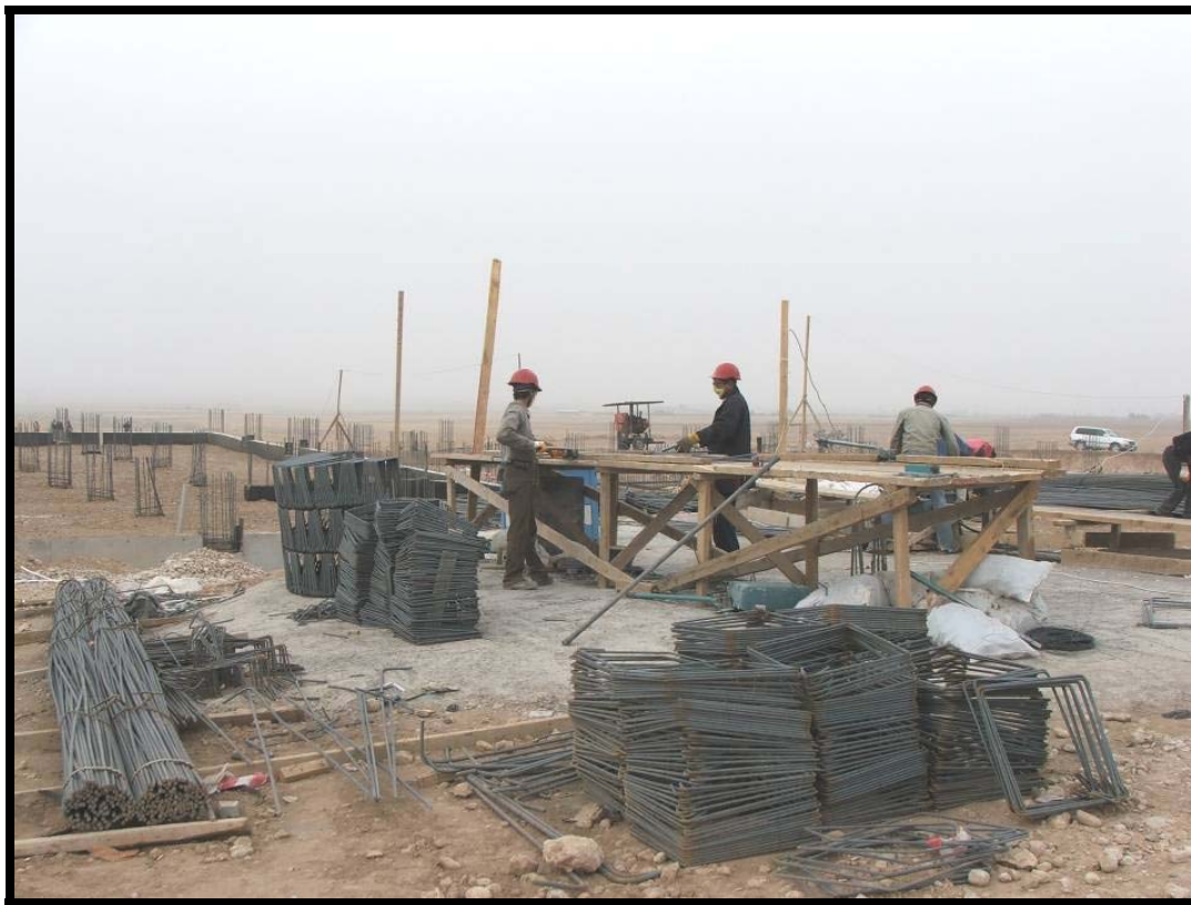
Site Photo 5. Workers used a bench with good equipment to measure, cut and bend rebar assembly sub-components used throughout the project.
