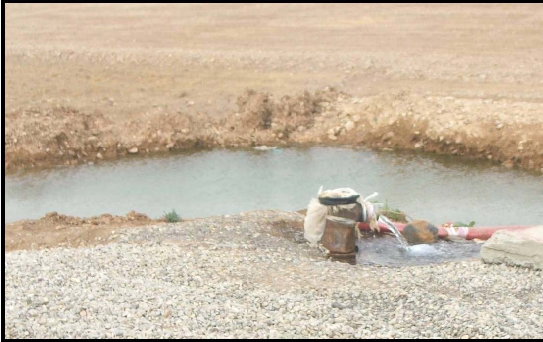
Site Photo 10. Ample clean water free flowed from both deep wells drilled on site.
