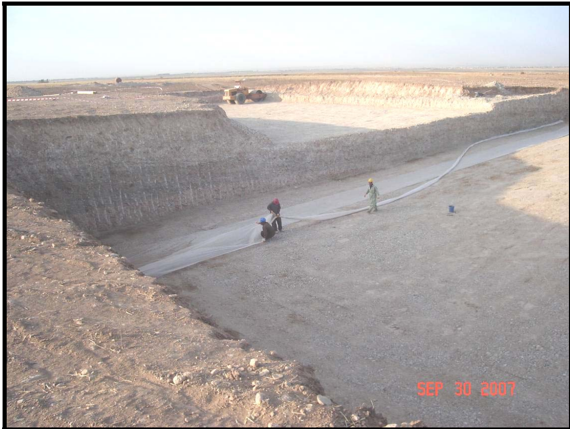
Site Photo 8. Pre-construction site preparation and excavation was extensive. (Photo courtesy of USACE)
