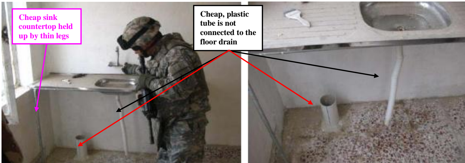
Site Photos 10 and 11. Examples of poor construction techniques by the contractor (Photos courtesy of the USACE)
