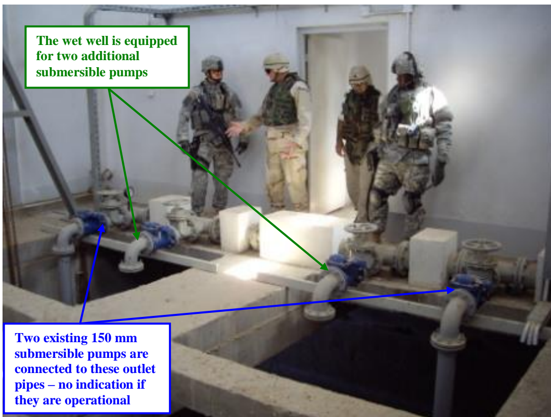
Site Photo 4. Interior view of Al Ghazaliyah G-6 building (Photo courtesy of the USACE)
