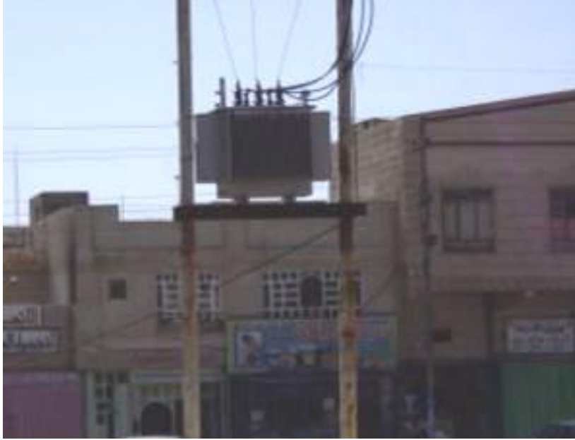
Site Photo 7. Transformer appears to be connected to main distribution grid (Photo courtesy of the USACE)
