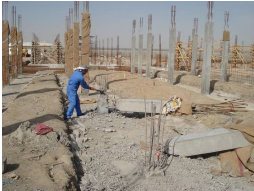
Site Photo 7. Removal of unacceptable concrete column shown in QA report dated 11 Feb 2008 (Courtesy of the USACE)
