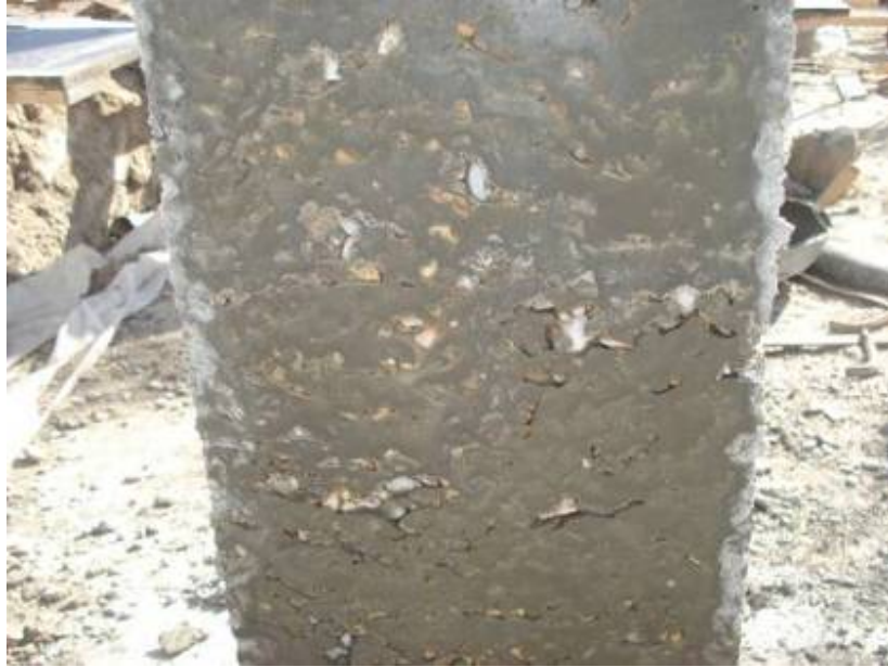
Site Photo 6. Concrete column segregation shown in QA report dated 7 Feb 2008 (Courtesy of the USACE)
