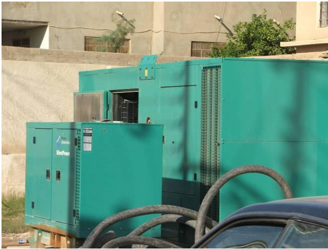
Site Photo 9. Backup generators
