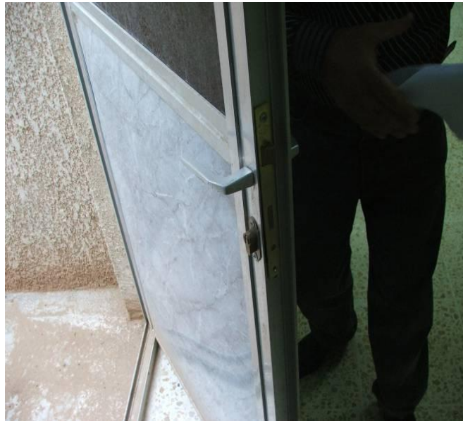
Site Photo 24. Low quality door latch
