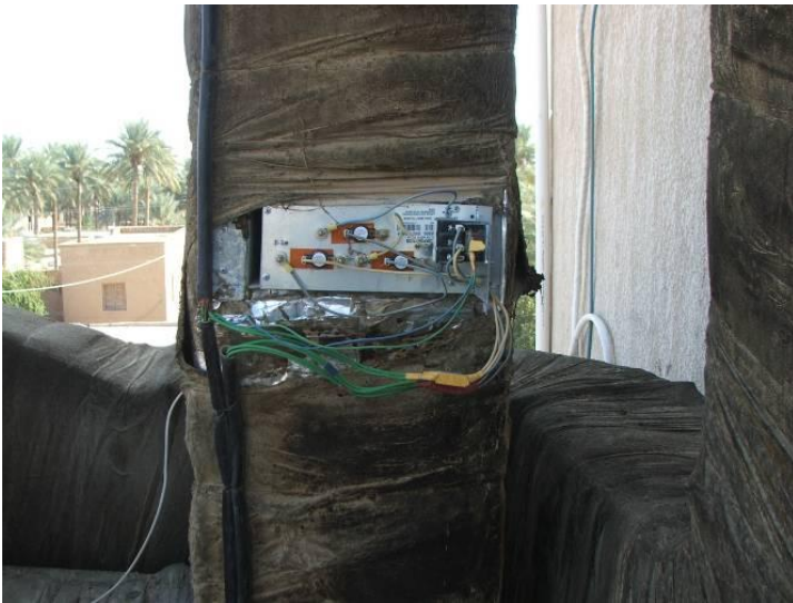
Site Photo 20. Unshielded damper
