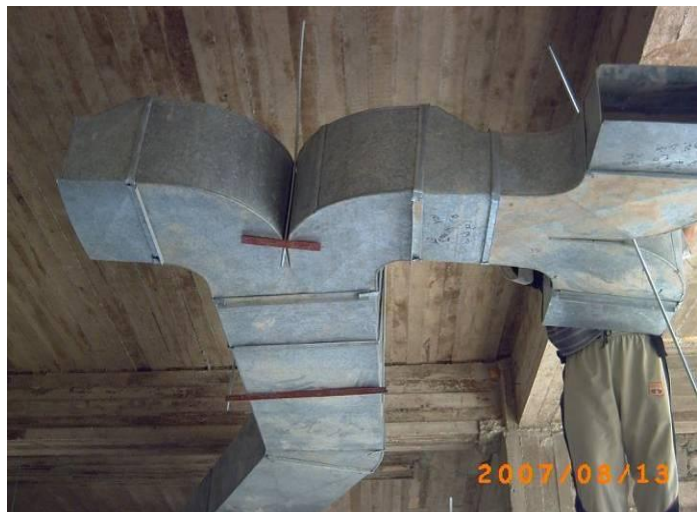
Site Photo 5. Interior HVAC ductwork (Courtesy of GRC)
