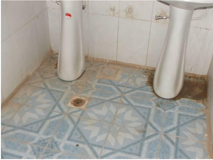
Site Photo 22. Leaking lavatory
