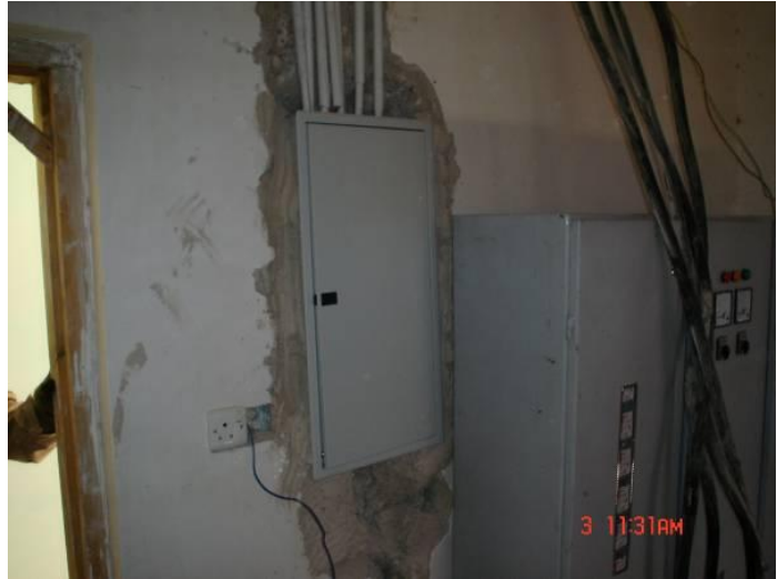
Site Photo 7. Main distribution panel (adequate electrical work) (Courtesy of GRC)
