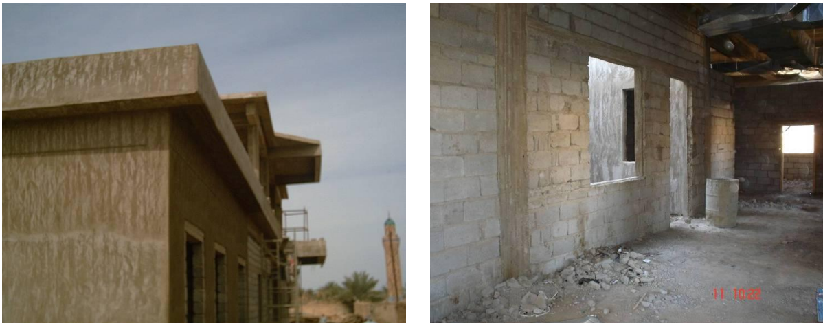
Site Photos 1 and 2. Interior and exterior views of the state of construction in March 2006 (Courtesy of GRC)
