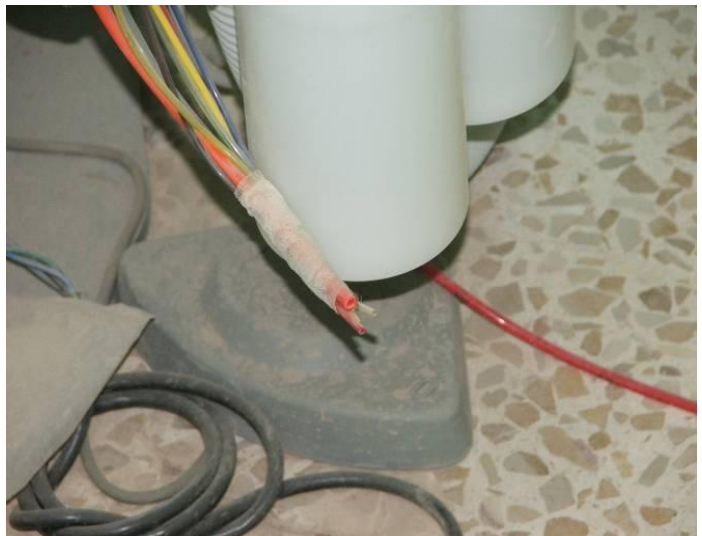
Site Photo 12. Disconnected utilities
