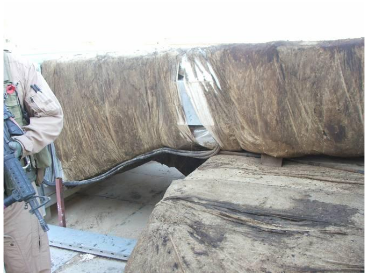
Site Photo 21. Duct insulation
