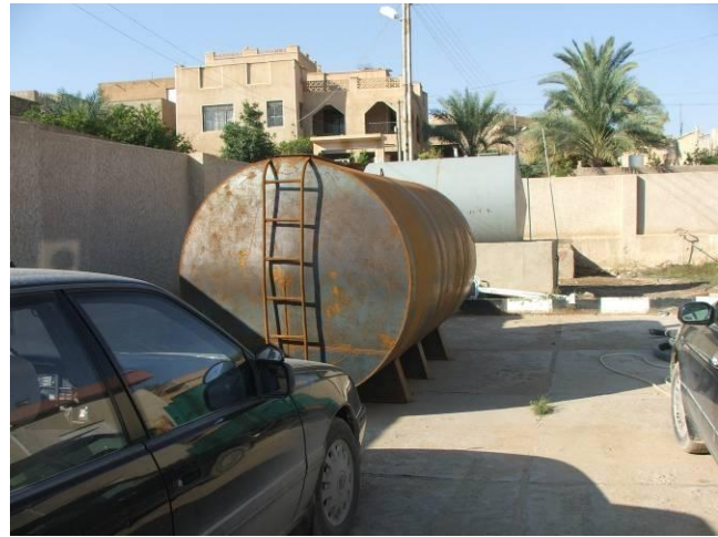
Site Photo 10. Fuel tank
