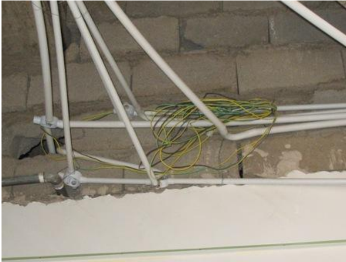
Site Photo 6. Example of poor electrical work (Courtesy of GRC)
