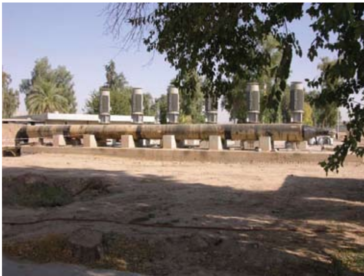
Dibbis Pump Station.
