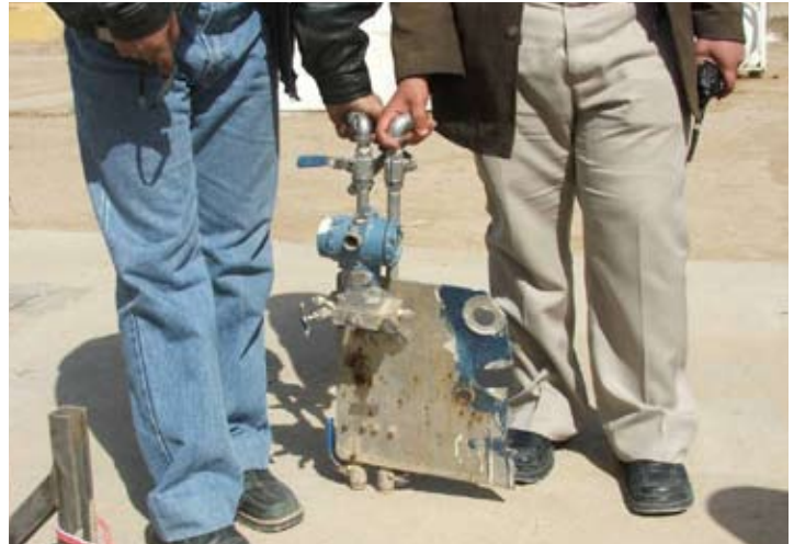
The disabled flow meter for the high-service pump-station meter vault.
