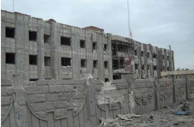
Damage to the north side of the services building and perimeter wall. (Photo courtesy of USACE)
