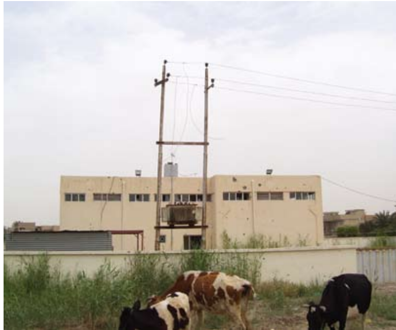
Iraq's electrical infrastructure remains in need of significant upgrade and repair.
