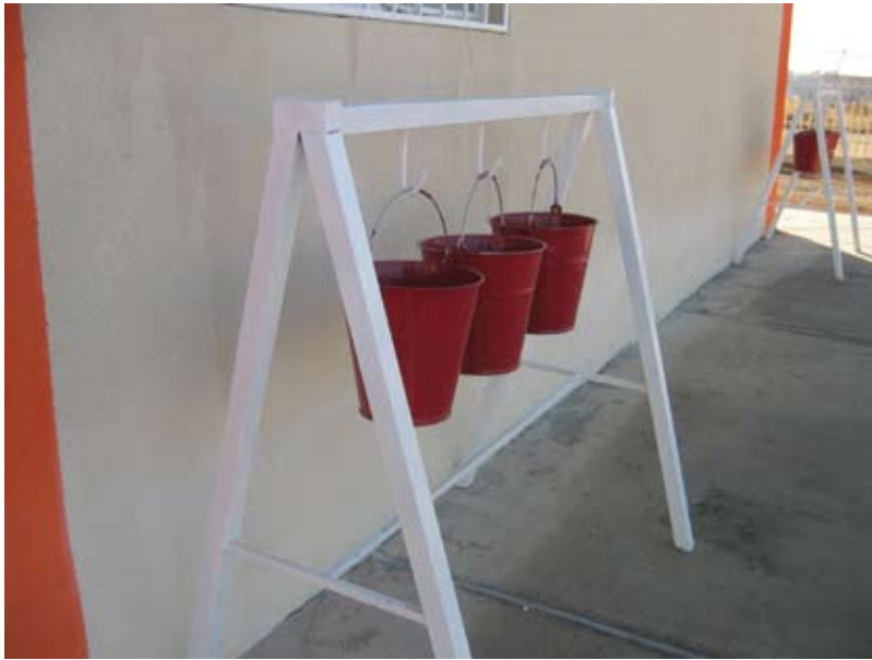
Fire-bucket racks, the only fire safety equipment observed at the time of the site visit.
