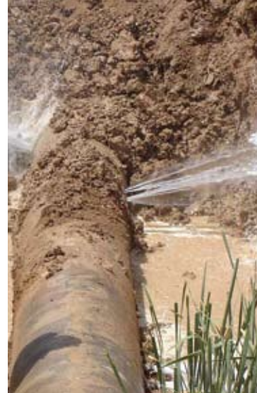
Example of leaks in the distribution lines throughout Iraq.
