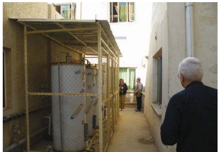
Water heaters placed between cadet barracks.
