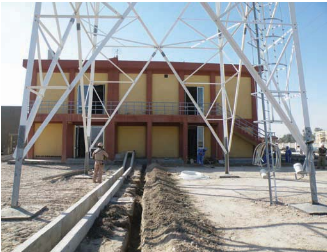
Cable trenches leading into substation building.
