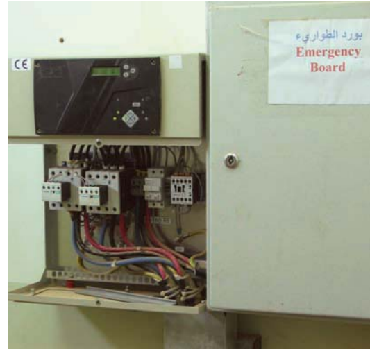
Access cover removed from non-functioning transfer switch.
