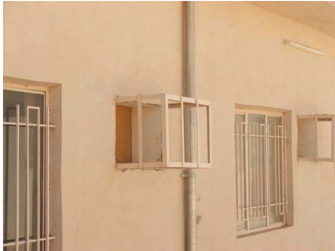
Installed air-conditioner mounts without units.
