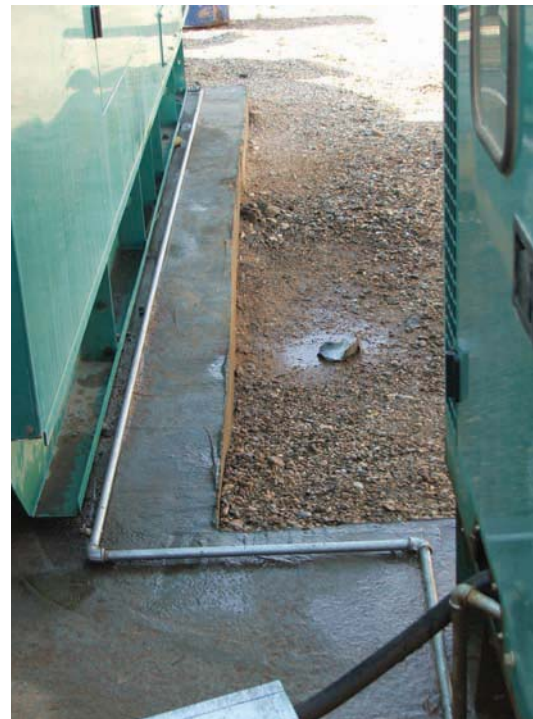
Diesel fuel spill and electrical line not installed correctly.
