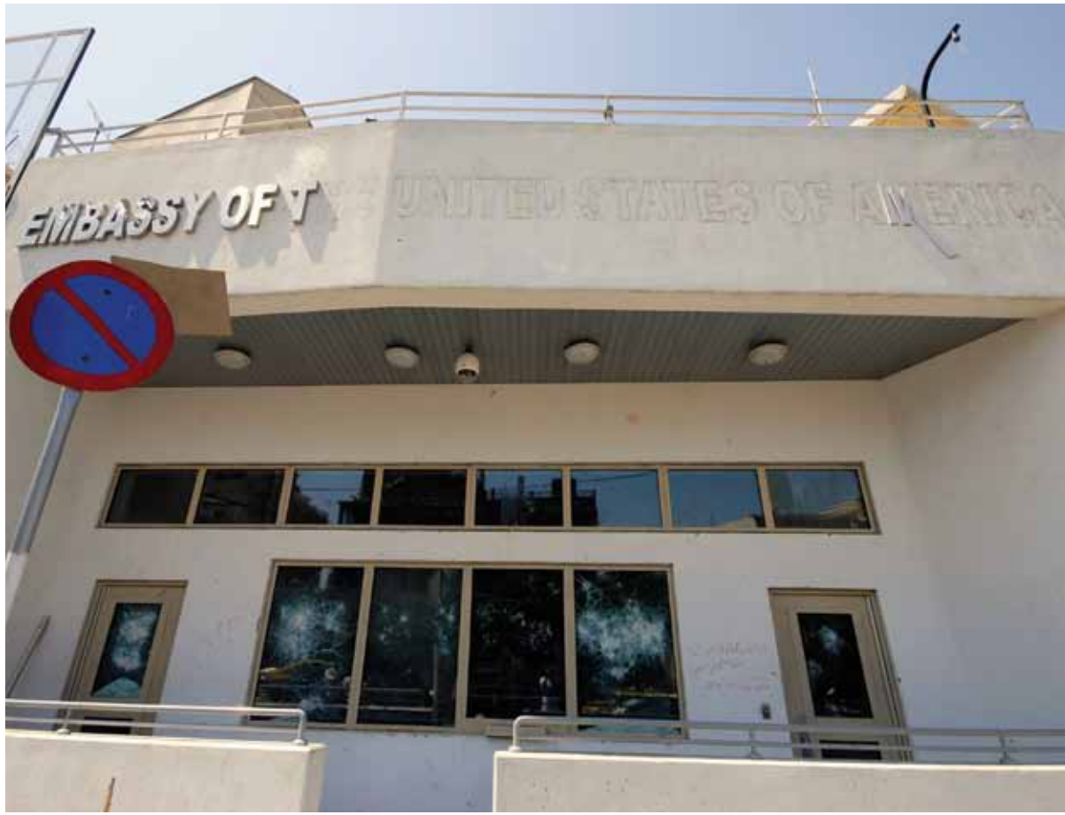
JULY 8 TO JULY 11 – DAMASCUS, SYRIA: ABOVE, THE FAÇADE OF THE U.S. EMBASSY REFLECTS DAMAGE INFLECTED BY DEMONSTRATORS WHO TORE AWAY MUCH OF THE SIGNAGE WHILE ASSAULTING THE BUILDING ON JULY 11, 2011. BELOW, A MAN CHECKS THE DAMAGED EXTERIOR OF THE COMPOUND. (AP/WIDE WORLD)
