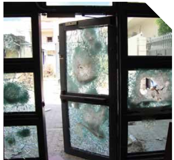
MAY 1 – TRIPOLI, LIBYA: THE BALLISTICS-RESISTANT GLASS INSTALLED IN THE DOORWAYS AT EMBASSY TRIPOLI'S CONSULAR OFFICES WITHSTOOD THE FURY OF AN ENRAGED LIBYAN MOB BEFORE FINALLY GIVING WAY TO INVADERS WHO TRASHED AND BURNT THIS AND OTHER BUILDINGS IN THE COMPOUND. (U.S. DEPARTMENT OF STATE PHOTO)
