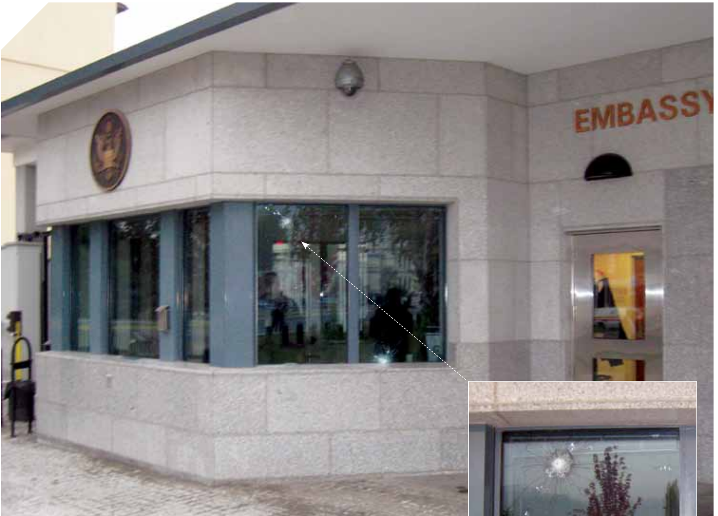
OCTOBER 28 – SARAJEVO, BOSNIA-HERZEGOVINA: GLASS AT THE FRONT OF EMBASSY SARAJEVO WAS CRACKED BUT NOT PENETRATED WHEN A GUNMAN ATTACKED THE BUILDING. (U.S. DEPARTMENT OF STATE PHOTO)
