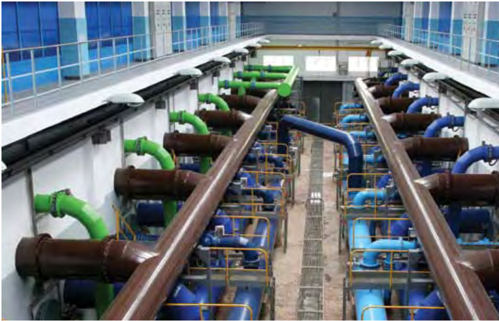
Interior of drinking water facility
