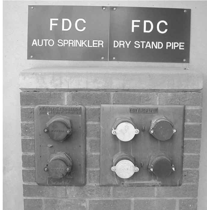
Figure 3-6 Preincident Planning Fire Department Connections Eliminate Confusion
