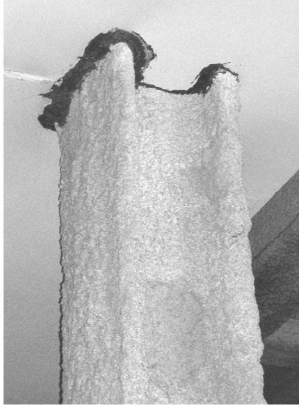
Figure 1-2 Spray-on fireproofing and smoke-seal caulking are two examples of passive fire protection.
