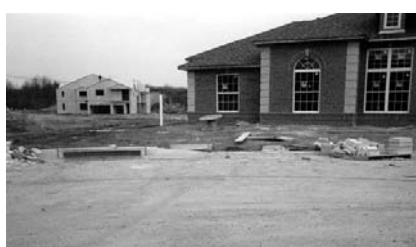
Improperly managed construction sites can clog estuaries with tons of sediments (photo by R. Ohrel).
