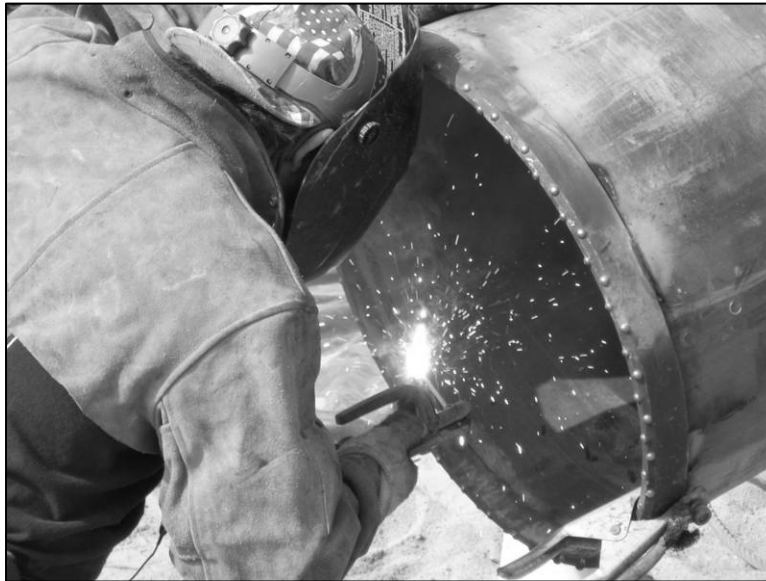
Photograph 3. Welding Caing shoe to the end of the 24-inch OD casing (February 4, 2006).
