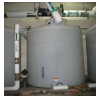
Large cisterns in the basement of EPA West collect rainwater as part of EPA's LID demonstration project.
