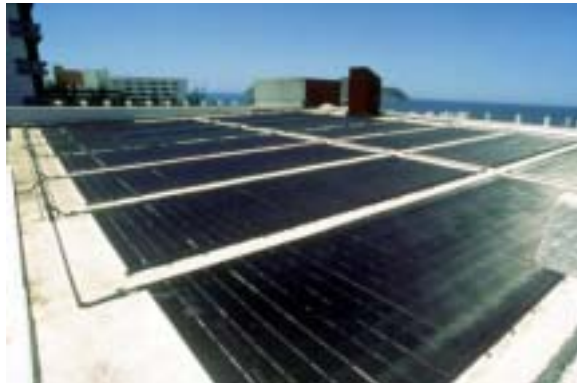
A solar heating system requires very little or no maintenance since it has no burners or moving parts. NREL/PIX08590
