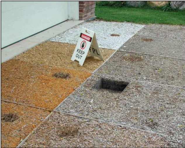
Figure 6—Removal of test sample for determination of density and moisture content of surface layer and EWF beneath surface.
