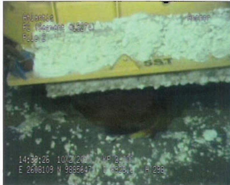
Figure 2.10 - P2 SCR Pile for Devil's Claw Connector from East Soil Scoured Approximate 0.5ft
