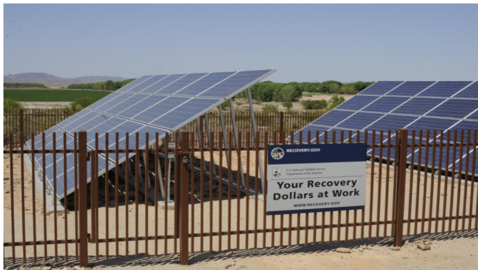
These solar panels at Cibola NWR (AZ) were installed with funds from the American Recovery and Reinvestment Act of 2009.
