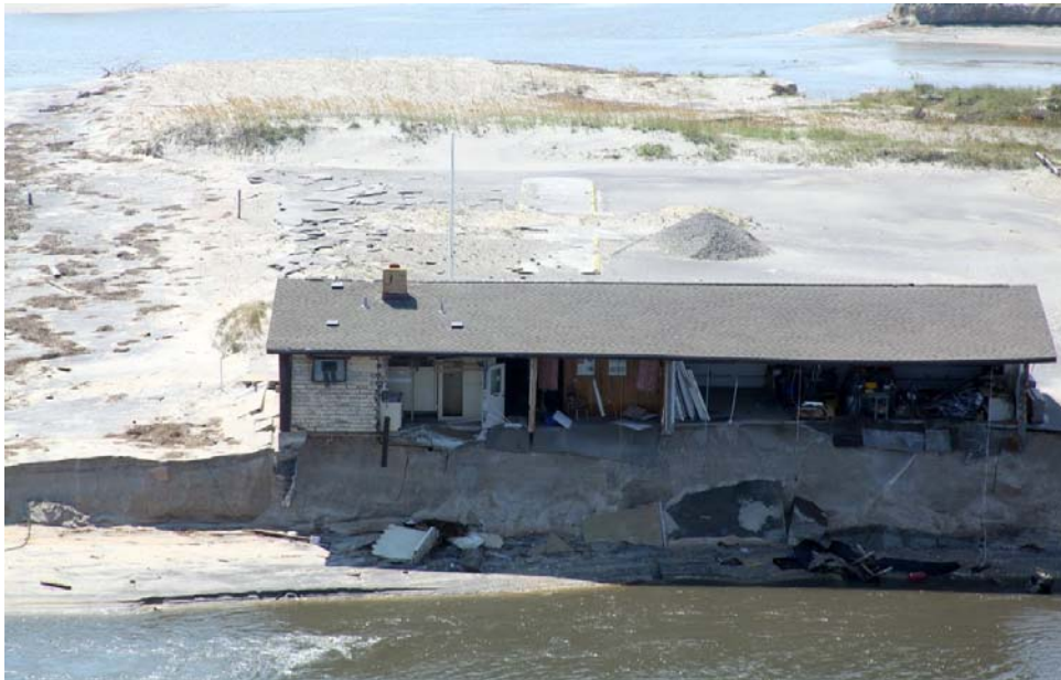
In recent years, natural disasters have added hundreds of millions of dollars to the deferred maintenance backlog. The above photo shows the destruction of a maintenance shop at Pea Island NWR (NC) from Hurricane Irene in 2011.
