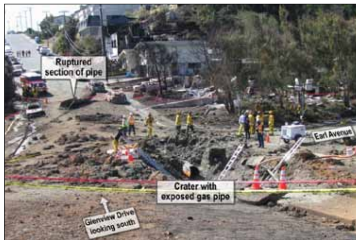
Figure 25. Ejected pipe section in San Bruno, California rupture and fire.
