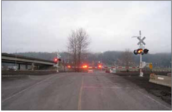
Figure 26. Longview active warning system.
