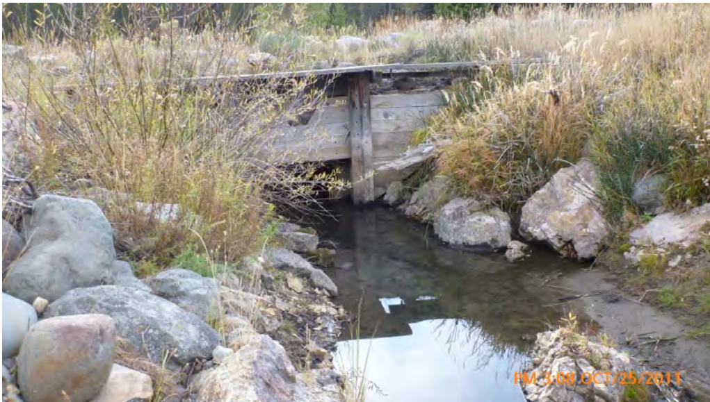
Photograph No. 42. View to the southwest looking downstream at the inlet of pond series three. Yankee Fork of the Salmon River, Yankee Fork Subbasin, Idaho – Bureau of Reclamation Photograph by P. Drury, October 25, 2011.
