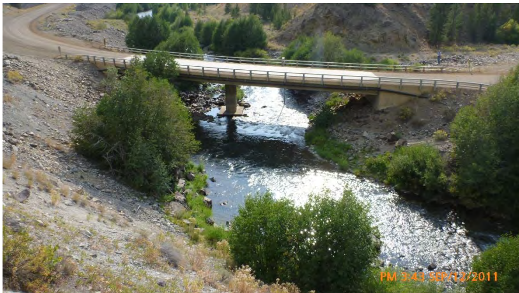
Photograph No. 14. View to the southwest looking downstream at a Custer Motorway bridge (Bonanza Bridge) crossing the Yankee Fork where the channel was constructed through dredge tailings in an area where the channel was naturally constricted by bedrock and colluvial deposits. Yankee Fork of the Salmon River, Yankee Fork Subbasin, Idaho – Bureau of Reclamation Photograph by P. Drury, September 12, 2011.
