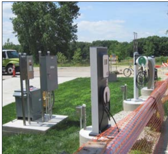
Figure 4. View of the EV charge stations of several different suppliers, installed by the Advanced Powertrain Test Facility.
