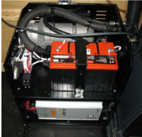
Figure 4. Battery Box Internal Components (compressor batteries & charger)
