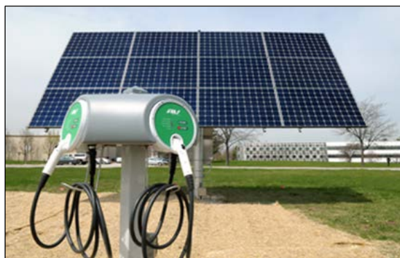
Figure 5. Argonne's solar energy array as a node for providing renewable solar energy for the pilot Smart Grid experiment to supply two vehicle charge stations.
