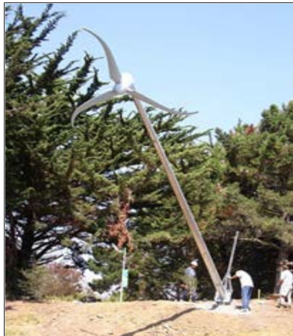
Figure 6. Installation of a wind turbine to provide another source of renewable energy connected to Argonne's pilot Smart Grid/EV Charging exercise.
