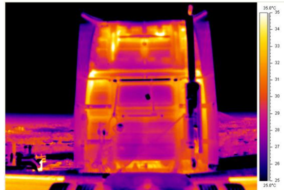
Figure 5. Infrared image of back exterior wall
