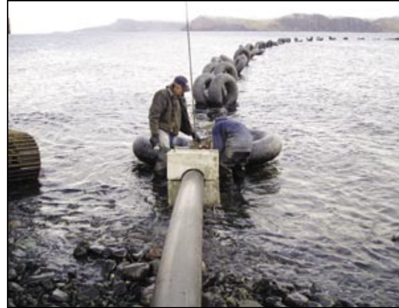
Figure 41: ANTHC Superintendent Al Gieske and local resident Matthew Bereskin install an ocean outfall line.
