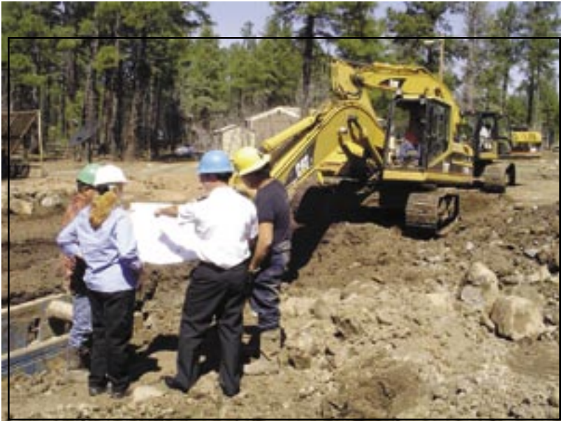
Figure 13: IHS engineers and technicians coordinate construction activities with the contractor as a sewer pipe is installed.
