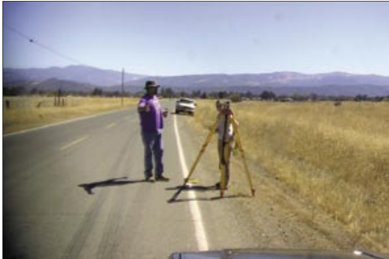
Figure 42: Engineer technician Tom Campbell and COSTEP Karla Secrist survey an 8-inch sewer main extension in California.
