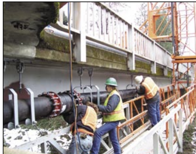
Figure 34: Bridge crossing installation of 10" ductile iron pipeline, California.
