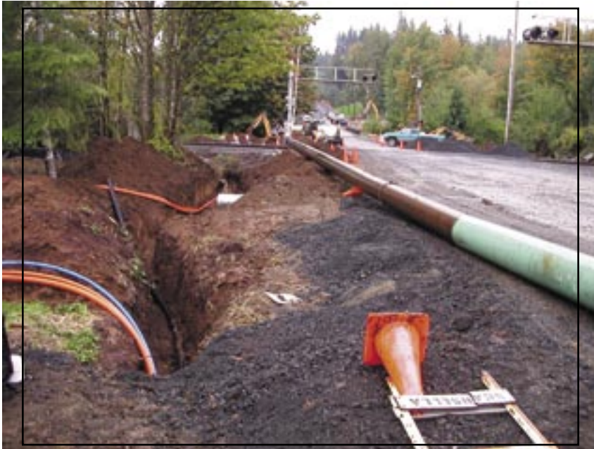
Figure 27: Railroad crossing casing.
