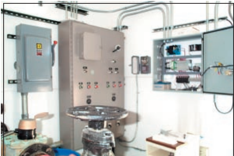
Figure 20: An automated controls system is being installed to control and monitor the water system and to allow operations control from the Utilities Department office.
