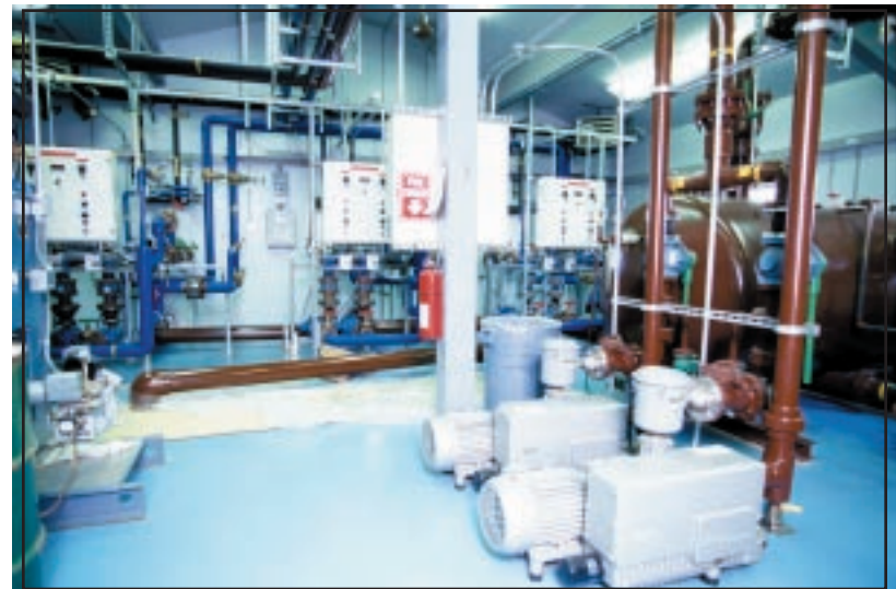
Figure 15: View of the sewage vacuum station equipment.
