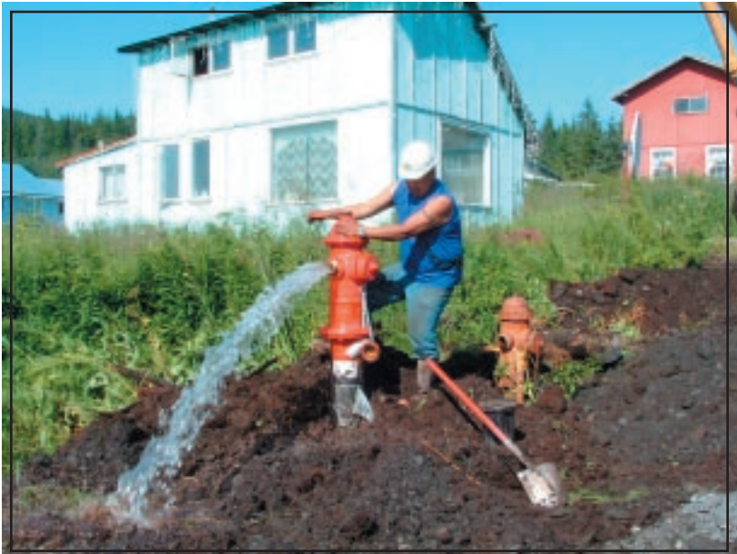
Figure 27: Gusty Wassillie, equipment operator, tests a newly installed fire hydrant. 1
