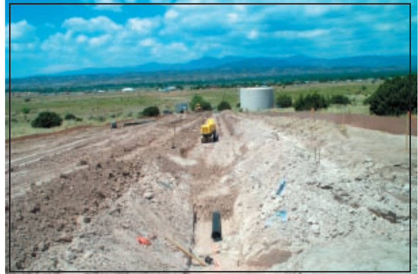
Figure 19: Trenching for the new waterline that will carry water to the new tanks.
