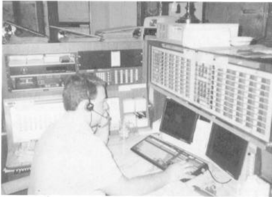
Exhibit 6-8. The consoles in the Montgomery County, Pennsylvania communications center were custom designed.
