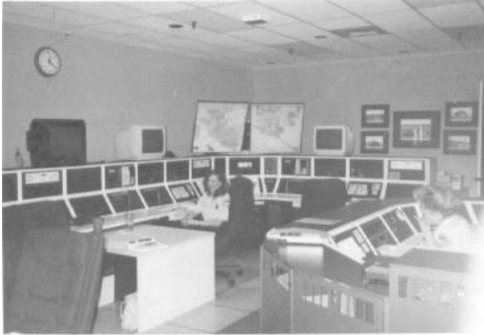
Exhibit 6-7. A commercially available radio control console installed in Huntington Beach, California.
