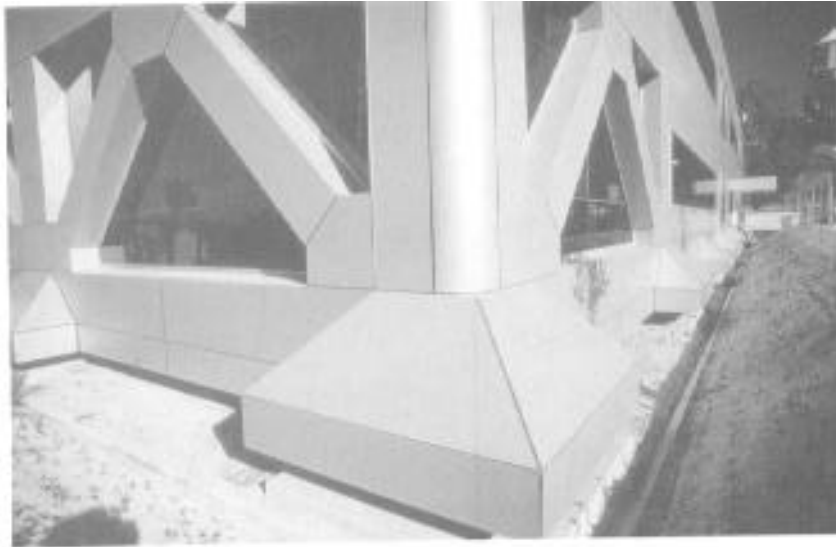
Exhibit 3-8. Detail of corner of L.A. County Command and Control facility. This corner (and the entire facility) is suspended on flexible base isolators.
