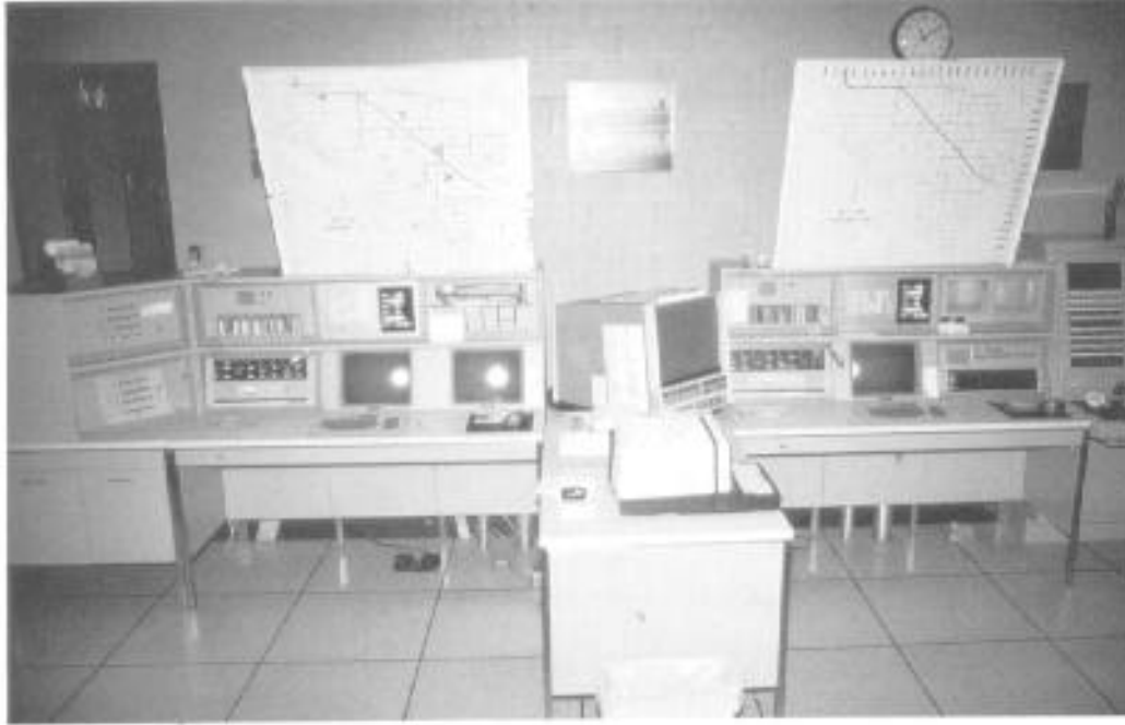
Exhibit 3-4. Huntington Beach, California, CAD System installed in the 1970s. The system has since been replaced.
