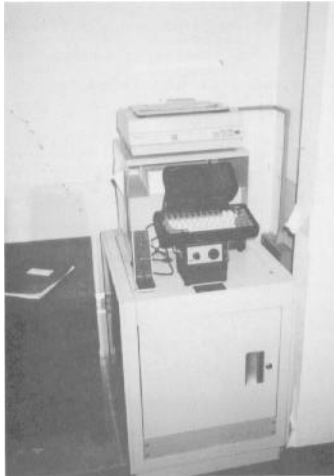
Exhibit 6-4. Fixed station radio in use at a fire station. Also note the printer, MDT, and external alarm used for redundant means of communication.
