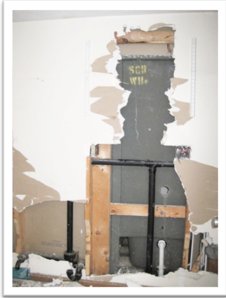
Figure 1: building stripped of plumbing pipes
