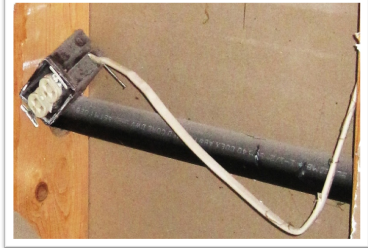
Figure 4: damaged wires leading to open electrical outlet
