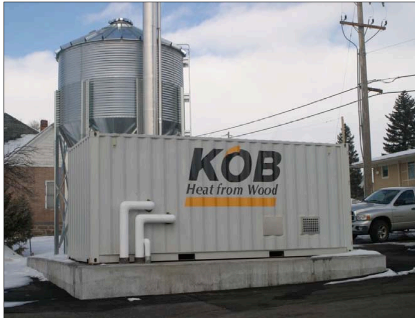
Figure 5. KÖB wood pellet boiler and pellet silo installed at Harney County District Hospital, Burns, Oregon Courtesy of A3 Energy Partners
